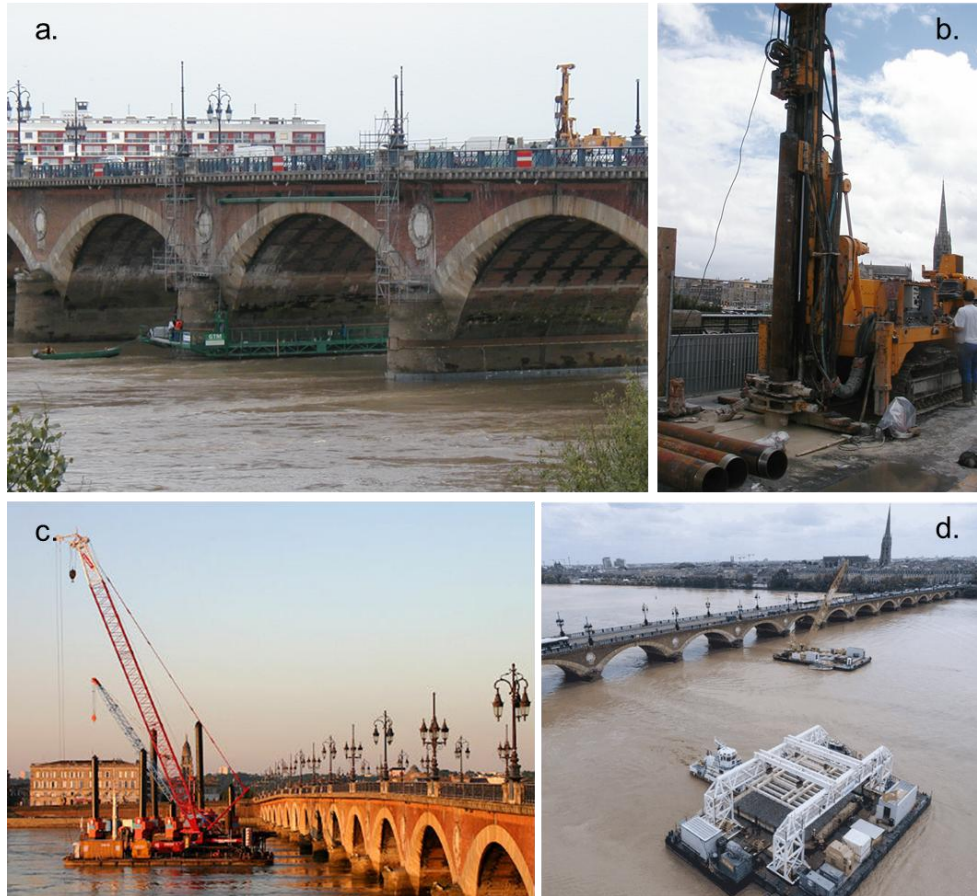
Figure 6. Illustration of works: (a) Post-tensioning on P05 and P06, (b) Micropiles on P05 and P06, (c) driven dolphins works on P08 and P09 (source: Bernard Tocheport), (d) rip-rap works on whole bridge (source: Sud-Ouest).
