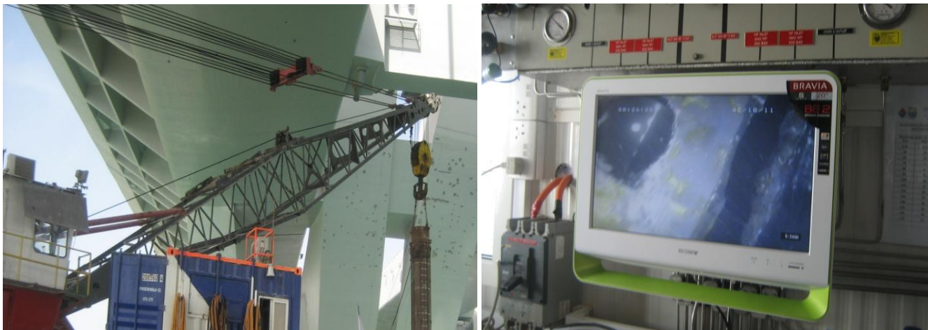
Figure 13. Casing Pile positioning inside an Existing Pile and view from the Diver's Screen.
