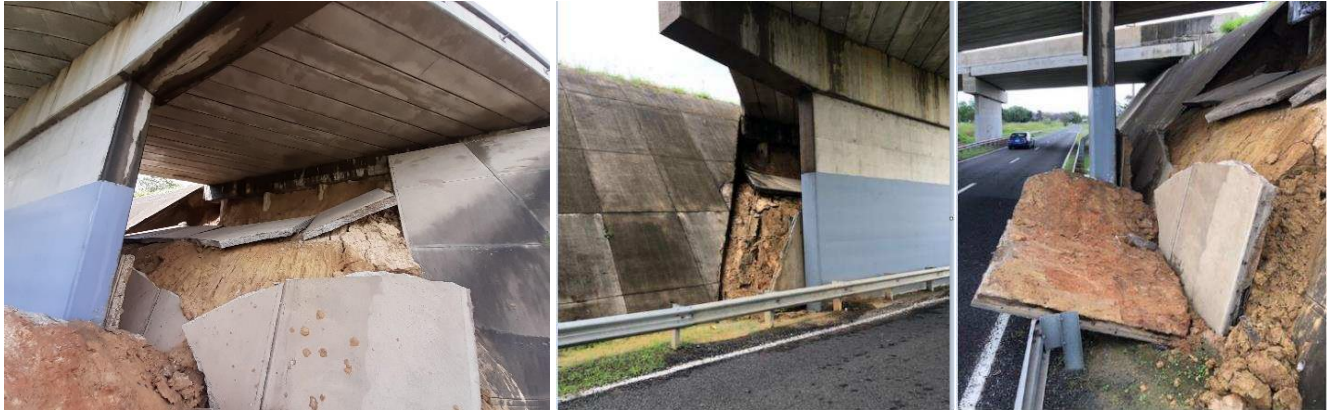
Figure 2. Abutment condition after failure.
