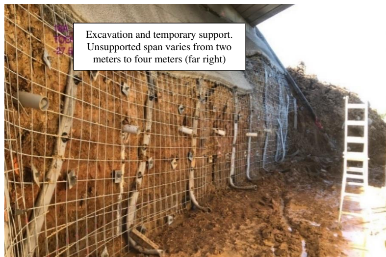
Figure 6. Excavation completed to formation level. The abutment is supported with percussion anchors and reinforced shotcrete. Note larger unsupported span on the far right.
