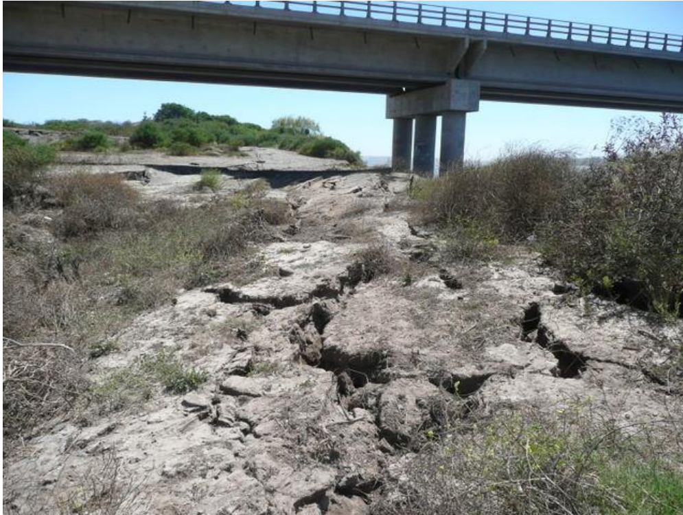
Figure 4. Liquefaction effects along the south side of the bridge (Bray et al., 2010).
