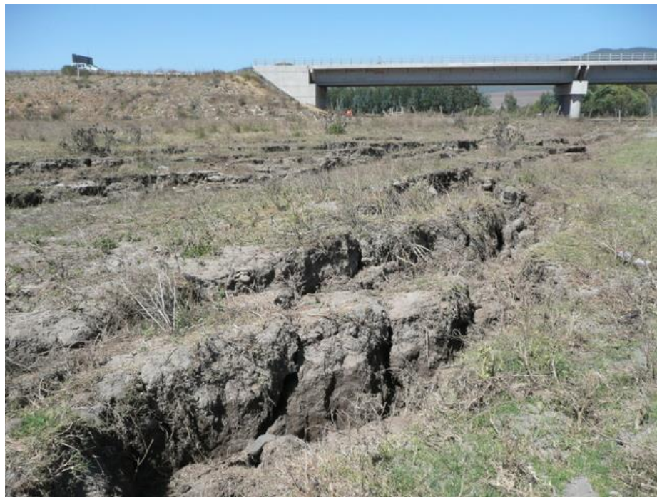
Figure 3. Lateral spreading at the north side of the bridge. Cracking showing roughly 0.6 m of vertical and 0.8 m of lateral displacement toward the river (Bray et al., 2010).
