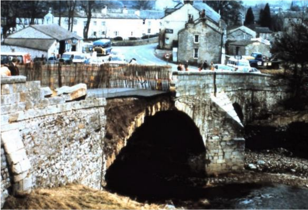
Figure 9. Failure of spandrel wall, Kettlewell New Bridge, 1984.
