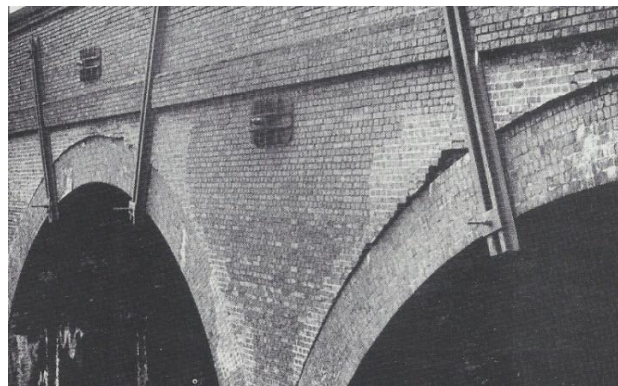
Figure 6. Tie-bars and spreader beams used to stabilize spandrel walls (Sowden and Jones, 1990).
