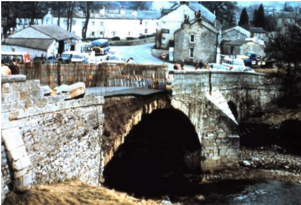
Figure 9. Failure of spandrel wall, Kettlewell New Bridge, 1984.
