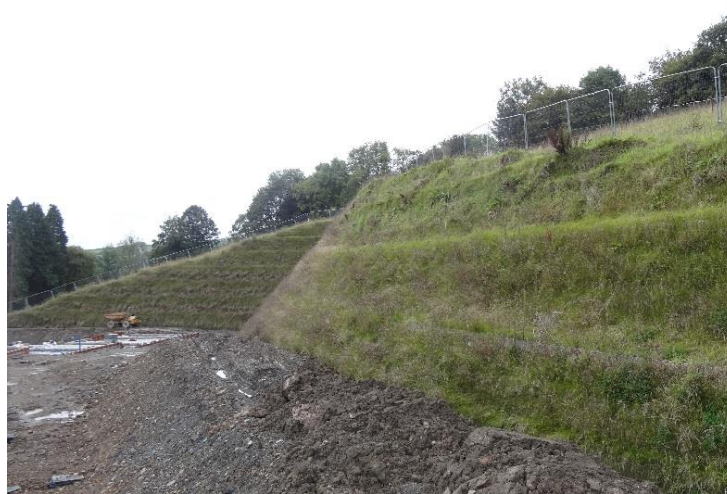
Figure 3. Vegetated structure constructed from draining geogrid and site won fill, Palmerston Park, Devon, Summer 2017.
