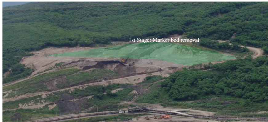
(a) Access road and Marker bed removal in 1 st Stage (as of August 2011)
