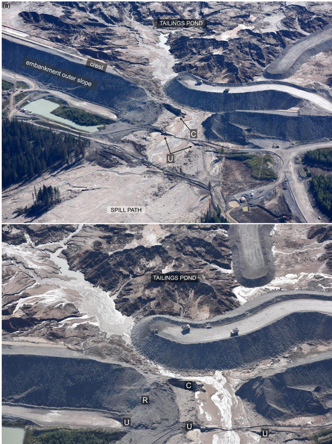
Figure 4. (a) Aerial diagonal view of the breach and spill path areas; (b) Aerial diagonal close-up of the breach location. Labels: C – core remnant, R – rockfill at the east boundary of the slide, U – uplift at the toe of the slide. Photography courtesy of Jamie Heath of terrasaurus.ca, taken 09/05/2014, reproduced with permission, altered to add labels.
