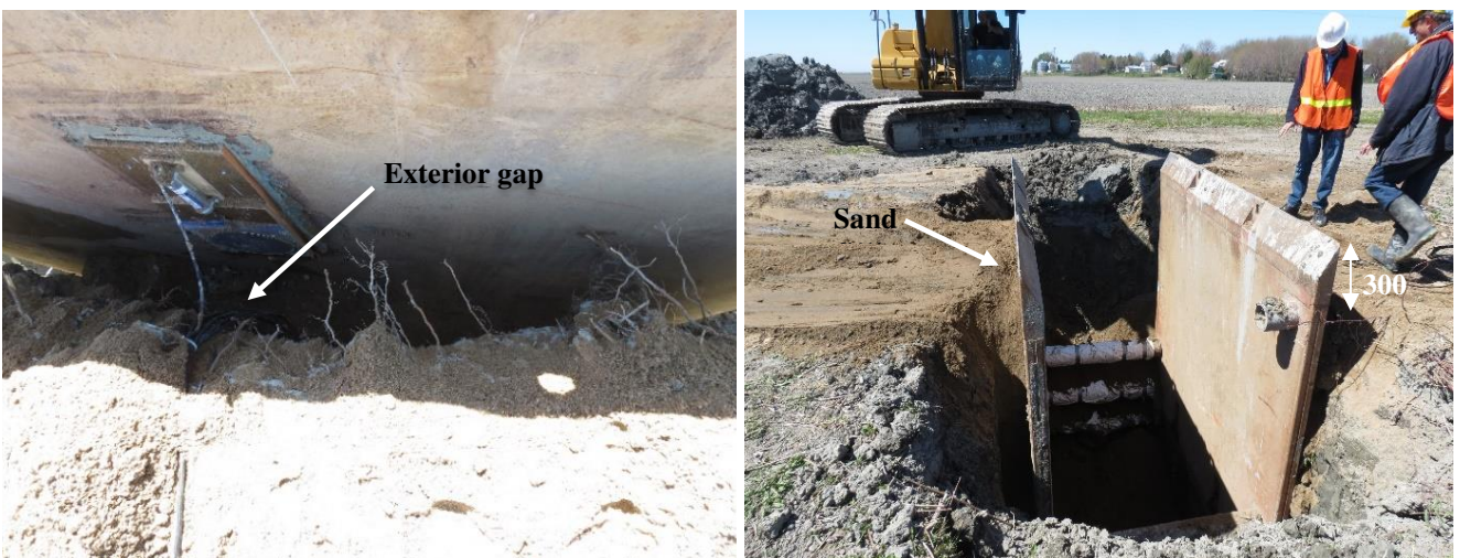
Figure 13. Sand was used to fill the space between the shoring exterior wall and the surrounding soil.
