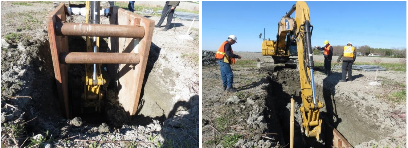
Figure 11. Excavation continued to make room to accommodate the second (upper) trench box in the trench.
