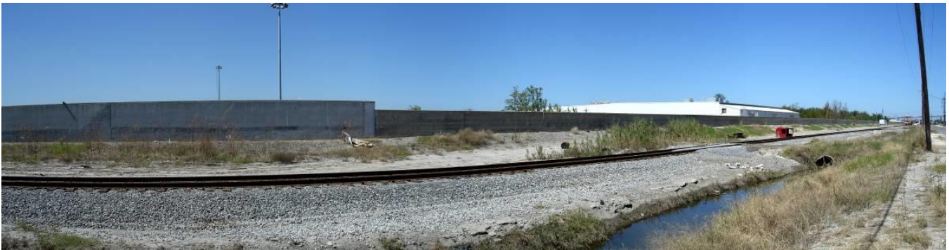
Figure 19. New L-wall and old I-wall transition near location of Katrina I-wall breach on IHNC West. (October 2, 2008, 29.9899° N, 90.0272° W)
