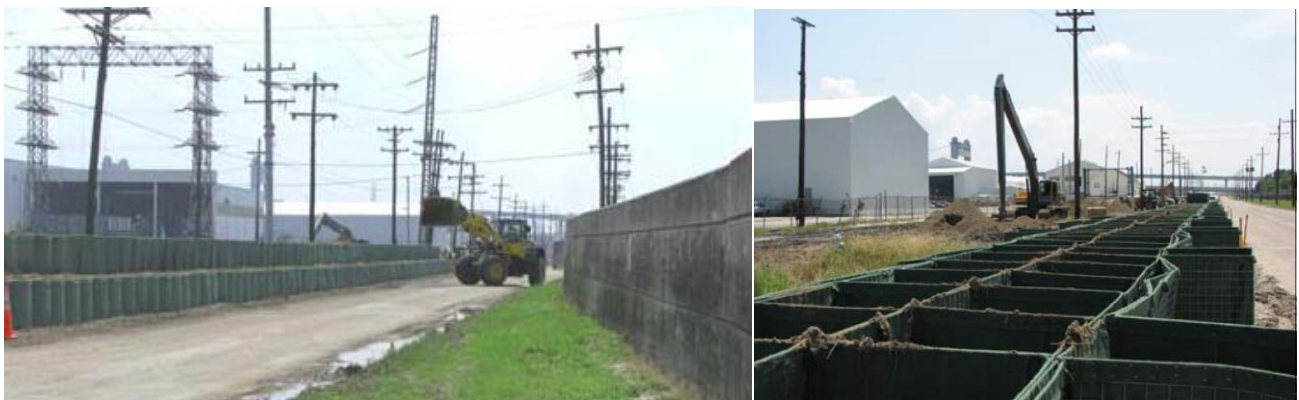
Figure 30. Temporary bin wall under construction, IHNC West along France Road. (August 2008, 30.0157° N, 90.0324° W, http://www.mvn.usace.army.mil/HPS/Status%20Report%20Newsletters/Sept_9_2008.pdf )
