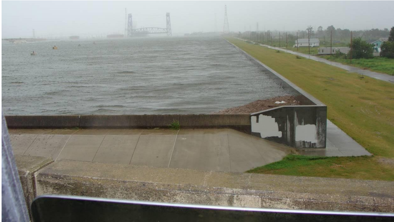
Figure 25. Gustav storm surge at IHNC East floodwall, taken from the Claiborne Avenue Bridge, looking north toward Florida Avenue Bridge (seen in background) from a perspective similar to that in Figure 18. (September 1, 2008, 29.9686° N, 90.0241° W, USACE)
