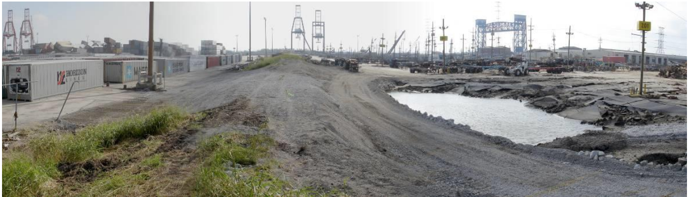
Figure 16. Post-Katrina IHNC West levee breach site, October 2005 (The breach had been temporarily repaired; note scour hole). (October 4, 2005, 29.9880° N, 90.0263° W, L. Wooten)
