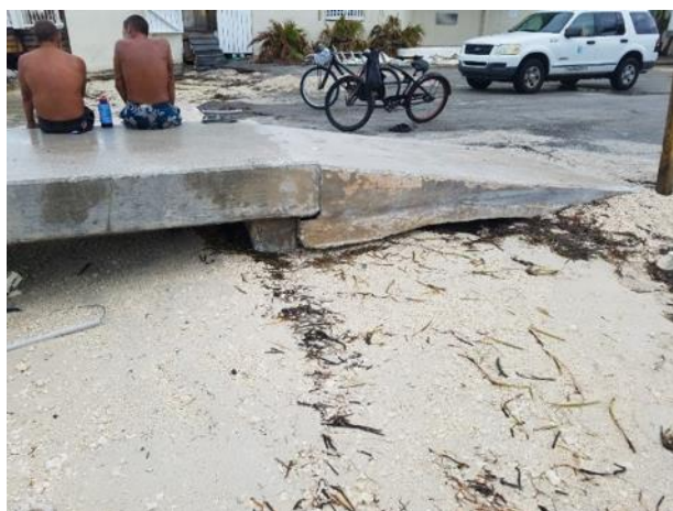
Figure 11. A concrete structure located on the eastern edge of Simonton Beach was undermined due to scour around the structure (collected September 27, 2017; location 24^{\circ}33'43.32''N , 81^{\circ}48'20.22''W ).
