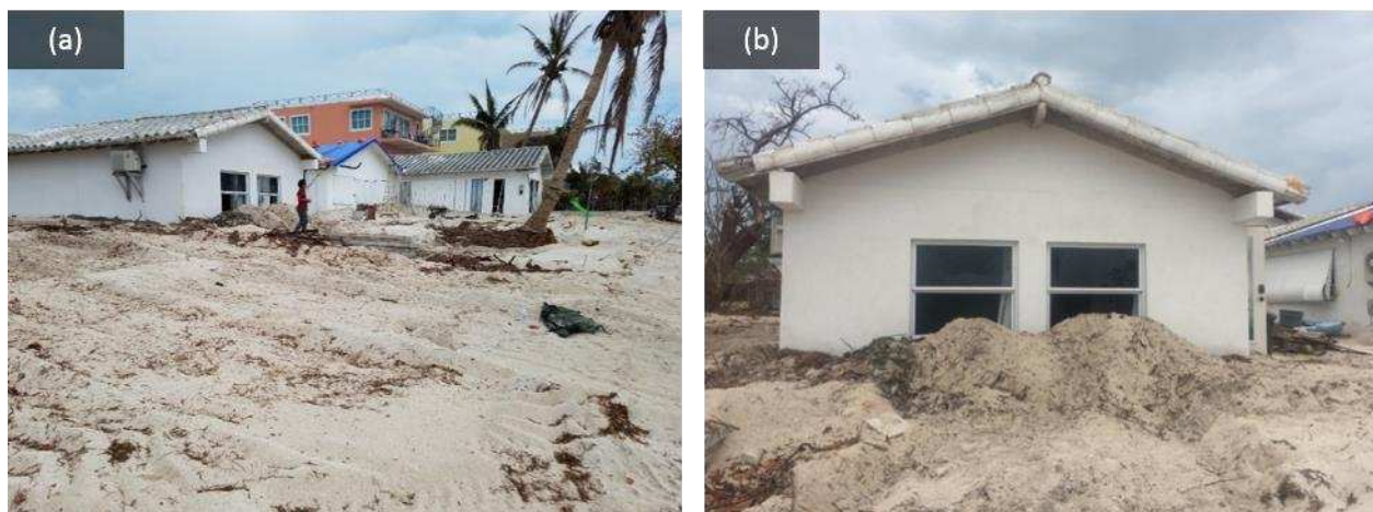
Figure 13. (a) Large volumes of sediment were deposited around houses and other structures and (b) buried them with approximately 1 m of sand, reaching the bottom of window sills (collected September 26, 2017; location 24°41'31.52"N, 81°4'56.31"W).
