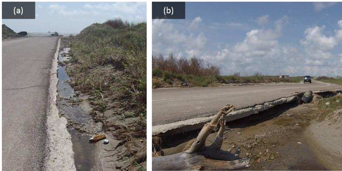
Figure 4. (a) Road undermining due to erosion and scour was observed on both sides of East Cotter Avenue, and (b) a 0.4 m undercut was measured at the beginning of a newly formed breach (collected September 3, 2017; location 27^{\circ}50'8.53''N , 97^{\circ}2'55.00''W ).
