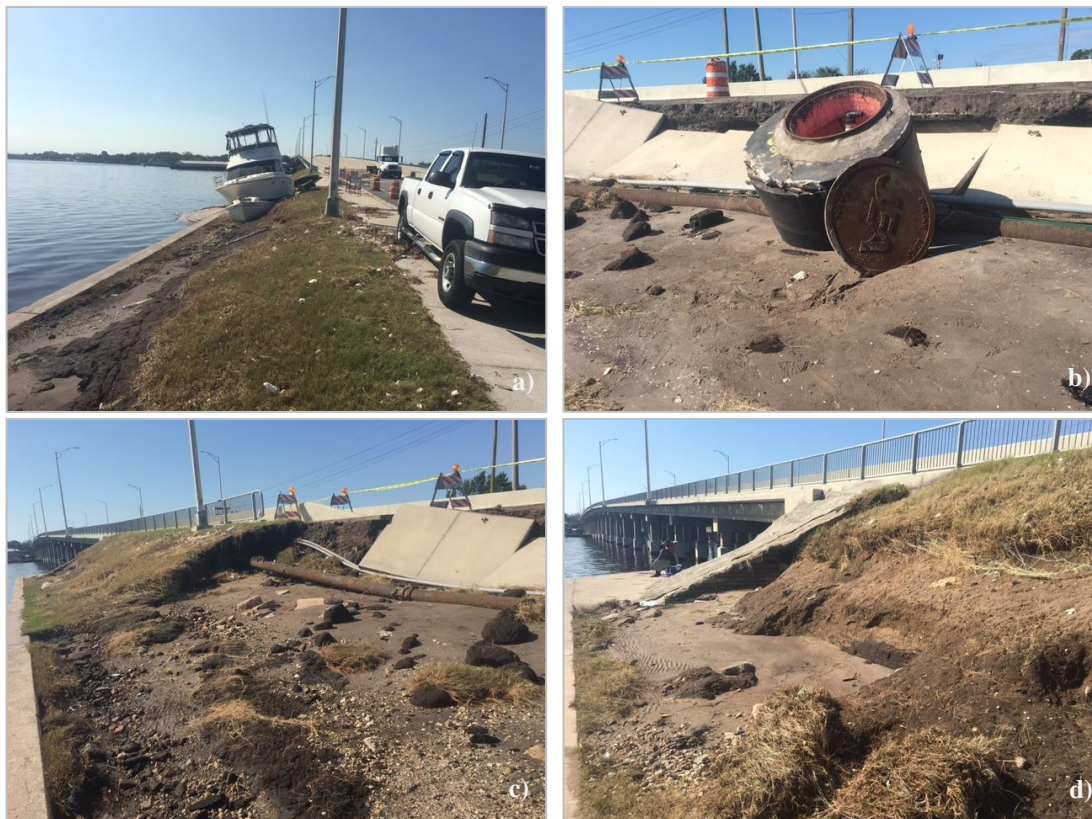
Figure 21. Erosion along the northeast embankment of the US 17 bridge over the Trout River at 30^{\circ}23'45.44''N latitude and 81^{\circ}38'53.95''W longitude shown from the north southward, including: (a) vessel washed ashore exacerbating scour, (b) an exposed sewer pipe and access structure, (c) exposed sewer pipe and electrical conduit and failed sidewalk, and (d) the terminus of scour at the stacked concrete sack wall where embankment cover was present (Hudyma et al., 2017).
