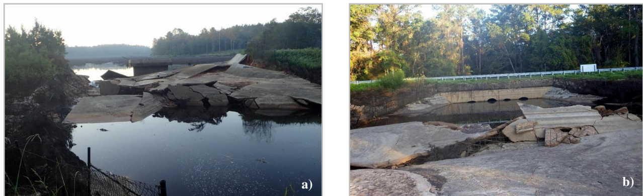
Figure 15: Failed Lake Hampton reservoir dam at 30°46'40.1"N latitude and 81°58'13.0"W longitude: (a) looking south from, and (b) looking north toward Lake Hampton Road.
