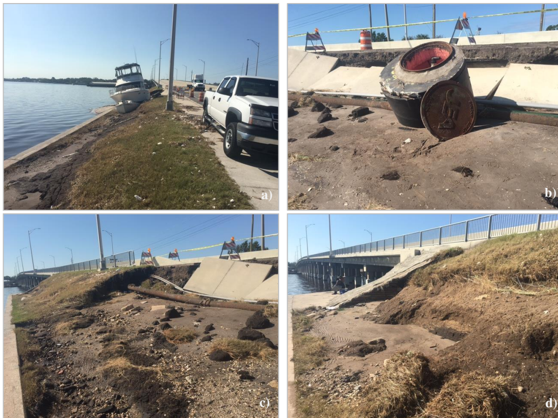
Figure 21. Erosion along the northeast embankment of the US 17 bridge over the Trout River at 30^{\circ}23'45.44''N latitude and 81^{\circ}38'53.95''W longitude shown from the north southward, including: (a) vessel washed ashore exacerbating scour, (b) an exposed sewer pipe and access structure, (c) exposed sewer pipe and electrical conduit and failed sidewalk, and (d) the terminus of scour at the stacked concrete sack wall where embankment cover was present (Hudyma et al., 2017).
