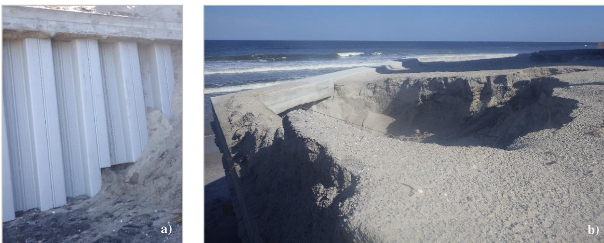
Figure 12: Sheet pile retaining wall failure from undercutting at 29°56'58.16"N latitude 81°18'11.96"W longitude, showing: (a) the exposed wall base, and (b) a funnel-shaped depression following basal soil escape (Hudyma et al., 2017).
