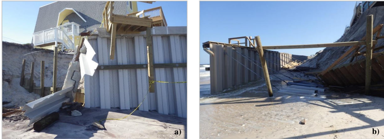
Figure 13: Failure of two residential sheet pile retaining walls from side erosion following Hurricane Irma, showing: (a) a partial sheet pile wing wall that was extended into the dune using timber piles and wooden lagging at 29^{\circ}56'55.10''N latitude and 81^{\circ}18'13.49''W longitude, and (b) the backside of the wall and anchors from the side where the wing wall was not yet installed at 29^{\circ}56'46.05''N latitude and 81^{\circ}18'7.5''W longitude (Hudyma et al., 2017).
