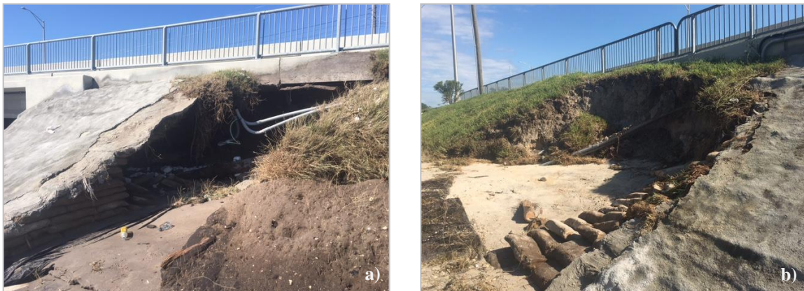
Figure 22. Scour damage along the (a) northeastern and (b) northwestern bridge embankment of the US 17 bridge over the Trout River at 30°23'44.43"N latitude and 81°38'54.13"W longitude (Hudyma et al., 2017).
