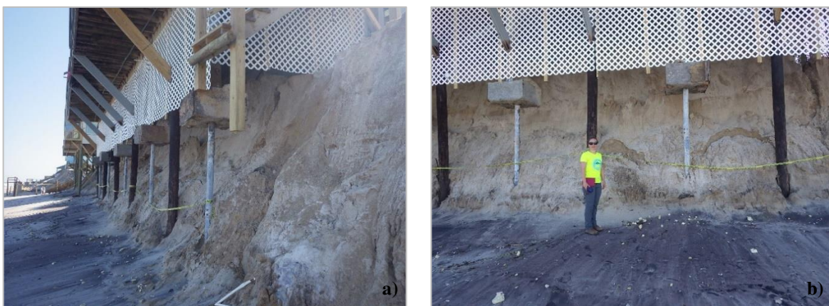
Figure 10: Erosion undercutting both the timber pile supports and micropile supported concrete footings for a beach house with continued slope failures in drying sand at 29°56'47.00"N latitude and 81°18'8.10"W longitude after Hurricane Irma.
