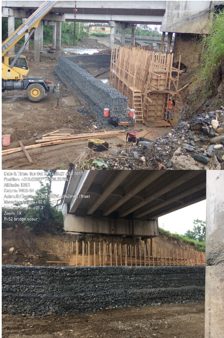
Figure 21: Photos of west abutment of westbound Highway 52 Bridge over the Inabón River (October 31, 2017; Silva-Tulla et al., 2018).
