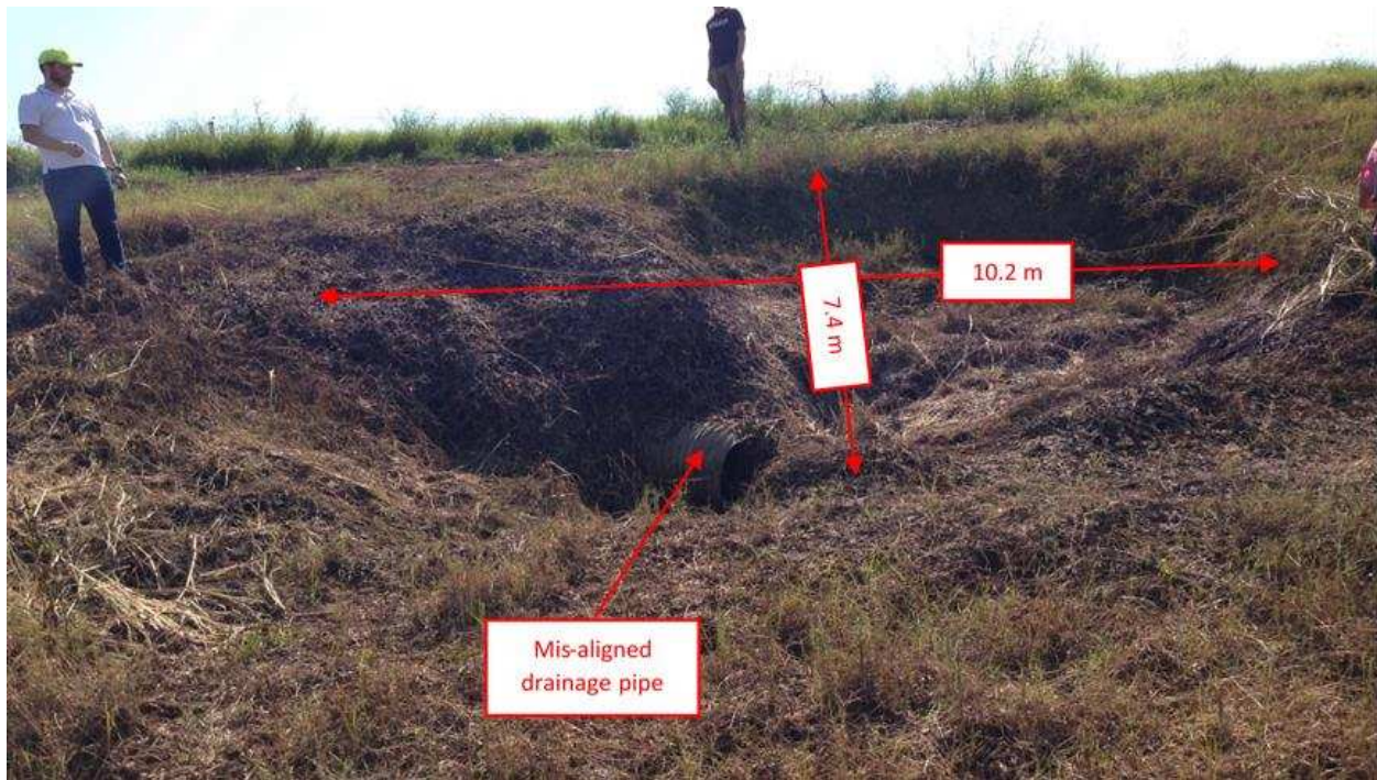
Figure 19. Sour hole at ruptured drainage pipe on Ditch H levee (September 10, 2017, 29.55759°N, 95.63768°W).
