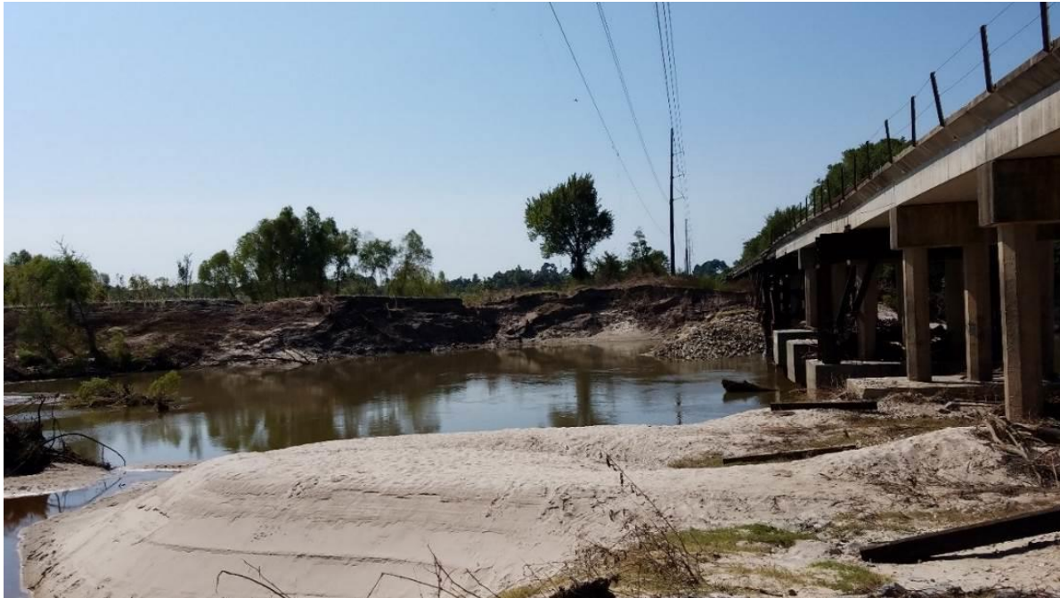
Figure 41. Bank erosion on the San Jacinto River downstream of I-45 and a railroad bridge parallel to the highway (September 11, 2017, Time 11:05 CDT, 30.24688° N, 95.45796° W).
