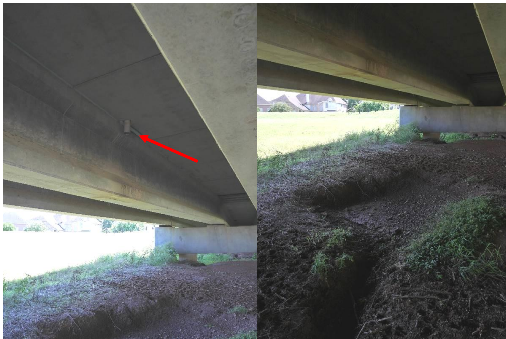
Figure 20. Erosion on Ditch H levee under the University Blvd Bridge due to flow impact from bridge drainage outfall (red arrow, September 10, 2017, 29.55902° N, 95.63744° W).
