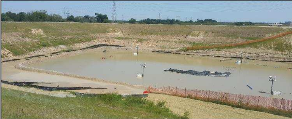
Figure 7. Interior of Addicks construction cofferdam for new outlet structure, flooded from Buffalo Bayou backwater; note erosion channels on slopes (September 9, 2017, 29.79063° N, 95.62586° W).
