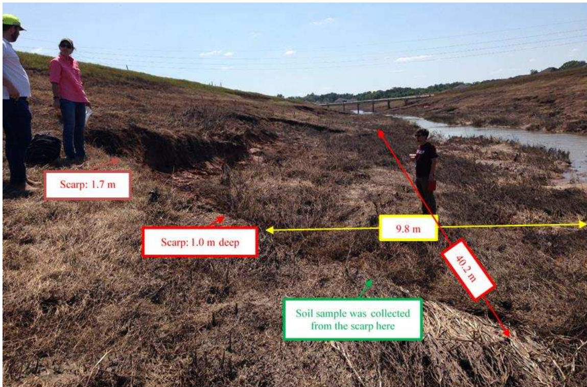
Figure 21. Slope failure north of damaged drainage pipe on the east side of ditch (September 10, 2017, 29.52647°N 95.56194°W),
