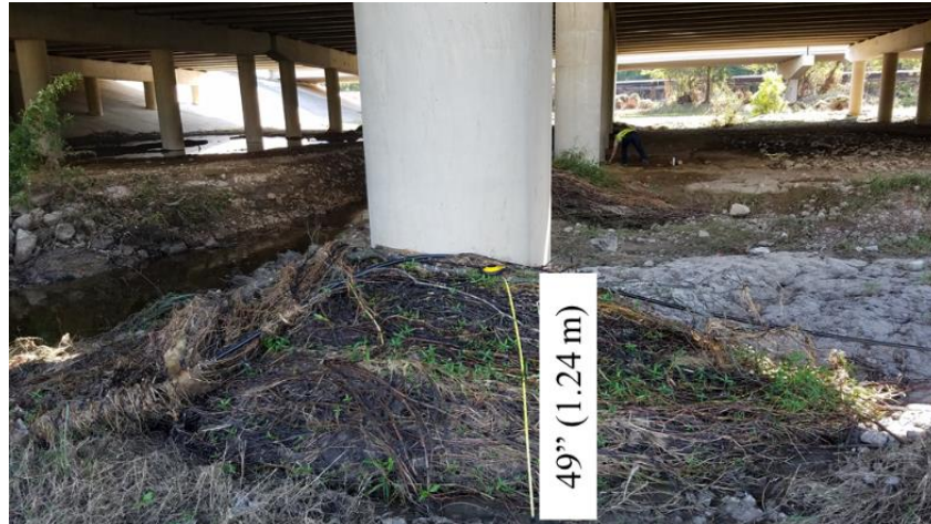
Figure 35. Observed debris on first column in flow direction. Debris pile is 1.24 m (49 inches) tall around the 1-m- (3-ft-) diameter bridge column (September 11, 2017, Time 10:04 CDT, 30.24688° N, 95.45796° W).
