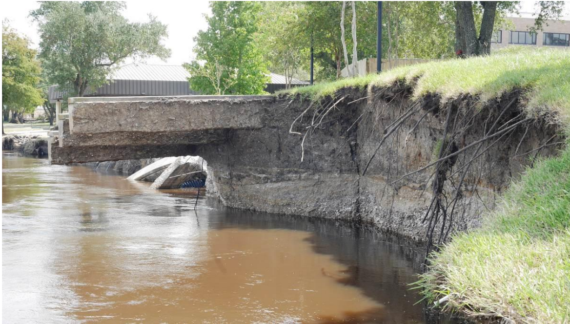
Figure 29. Scour under amphitheater structure. Scarp is estimated to be about 12 m (40 ft) back from previous shoreline (September 11, 2017, 30.08334° N, 94.09441° W).
