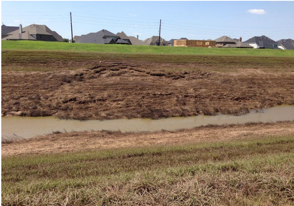
Figure 22. Earth slumping on the west side embankment (September 10, 2017, 29.53103° N, 95.56200° W).
