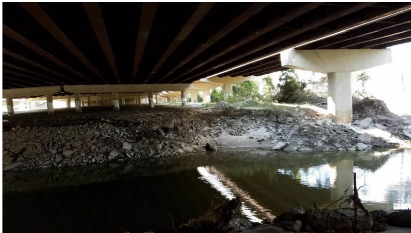
Figure 39. Riprap along south bank of San Jacinto River (September 11, 2017, Time 10:56 CDT, 30.24574° N, 95.45761° W).
