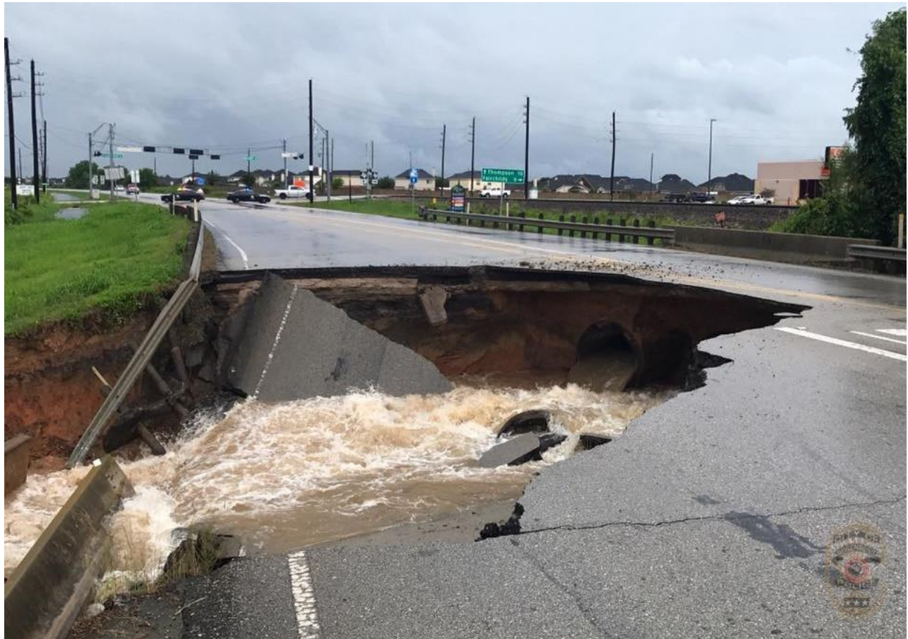
Figure 43. FM 762 Washout on August 27, 2017 (Courtesy of the Rosenberg Police Department, 29.5442° N, 95.7434° W).
