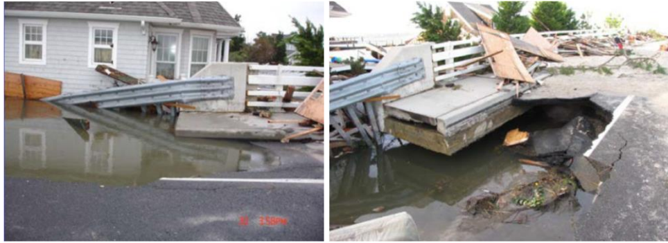
Figure 11. Mantoloking Bridge east abutment erosion (40.040058°N, 74.051886°W, Ocean Ct. Eng., 2012; GEER, 2014).
