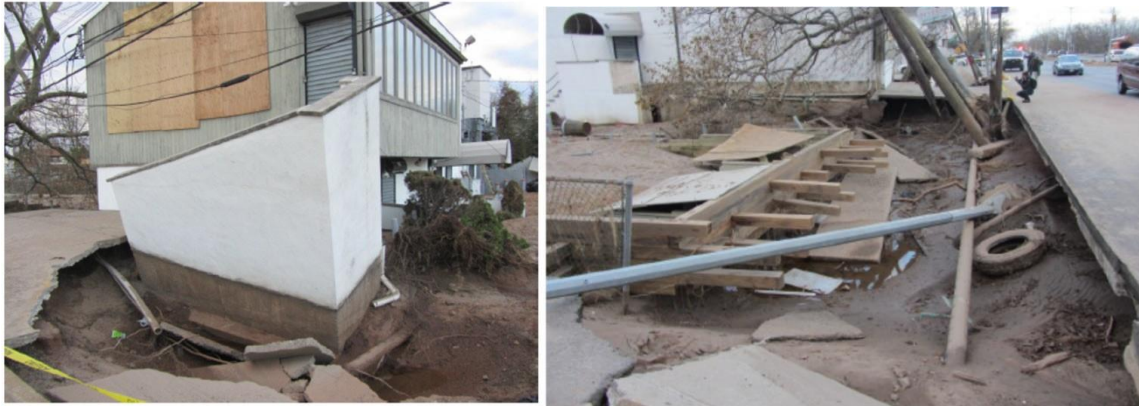
Figure 23. Scour undermining at Seaver Ave & Father Capodanno Blvd, SI (40.575944° N, 74.083015° W, 11/4/12). Damage to stair foundation and drain (left) and sidewalk, utilities, and light pole foundation (right). Photos by GEER (2014).
