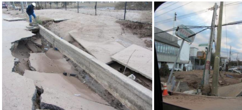
Figure 24. Scour undermining of street and utilities at Seaview Blvd, SI (40.579283°N, 74.077849°W, 11/4/12, GEER, 2014).
