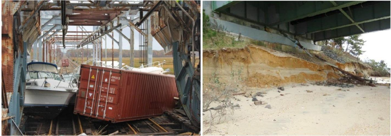
Figure 8. Morgan Drawbridge (left; NJ Transit) and Rt. 72 abutment erosion, looking south-east (right; NJDoT).
