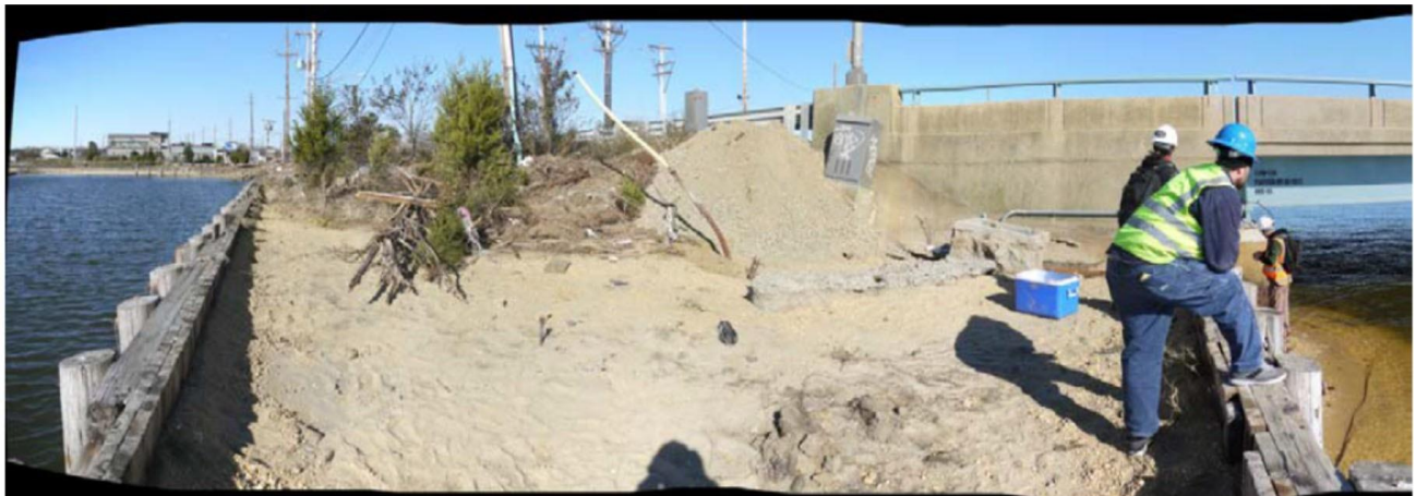
Figure 9. Erosion at Mathis Bridge southwest abutment (eastbound Rt37) ( 39.949350^{\circ}\text{N} , 74.113902^{\circ}\text{W} ; GEER 2014).
