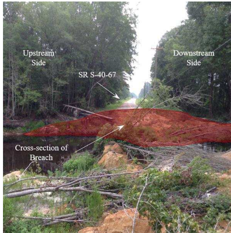
Figure 6. Cross-sectional area of breach in Dam A (east view from SR-40-67).
