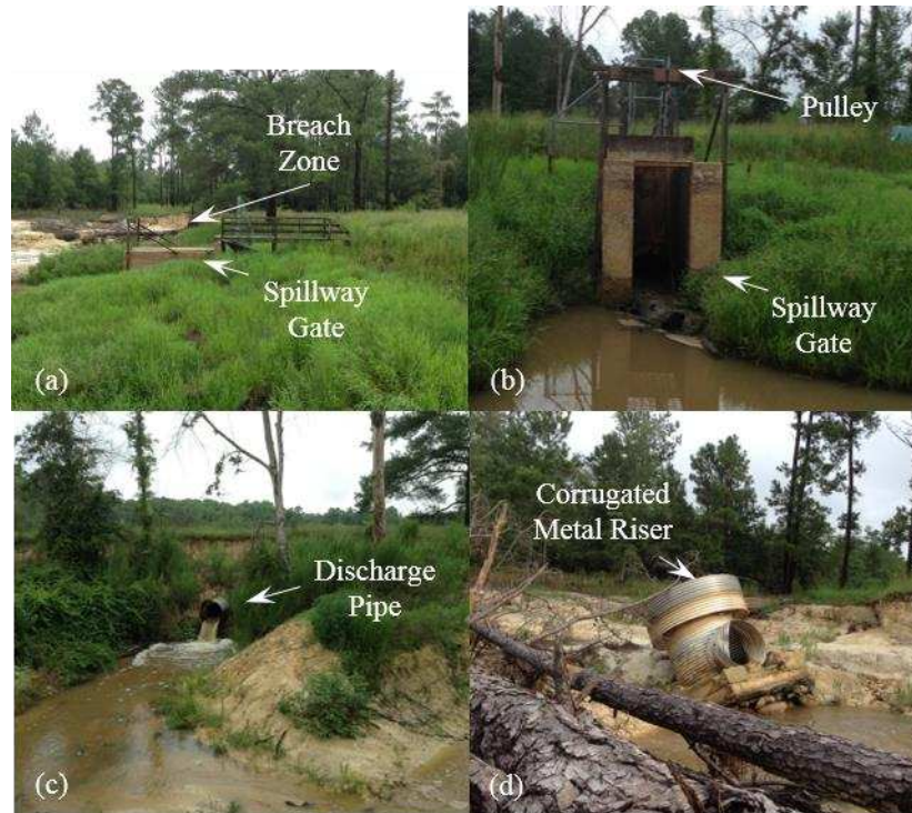
Figure 14. Spillway structures in Dam B: (a) location (view along the crest looking north), (b) concrete spillway gate (east view from upstream), (c) discharge pipe downstream from gate (east view from downstream), and (d) failed riser (northwest view from breach).
