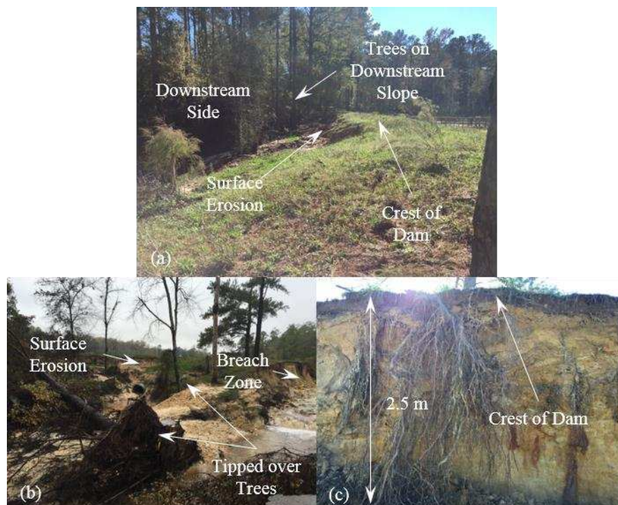
Figure 15. Vegetation on Dam B: (a) low grasses and small bushes on the dam crest, trees on downstream side slope (south view from crest), (b) tipped over trees near breach and zone of surface erosion (west view from downstream), and (c) presence of roots throughout the dam on the south breach wall (south view from breach).
