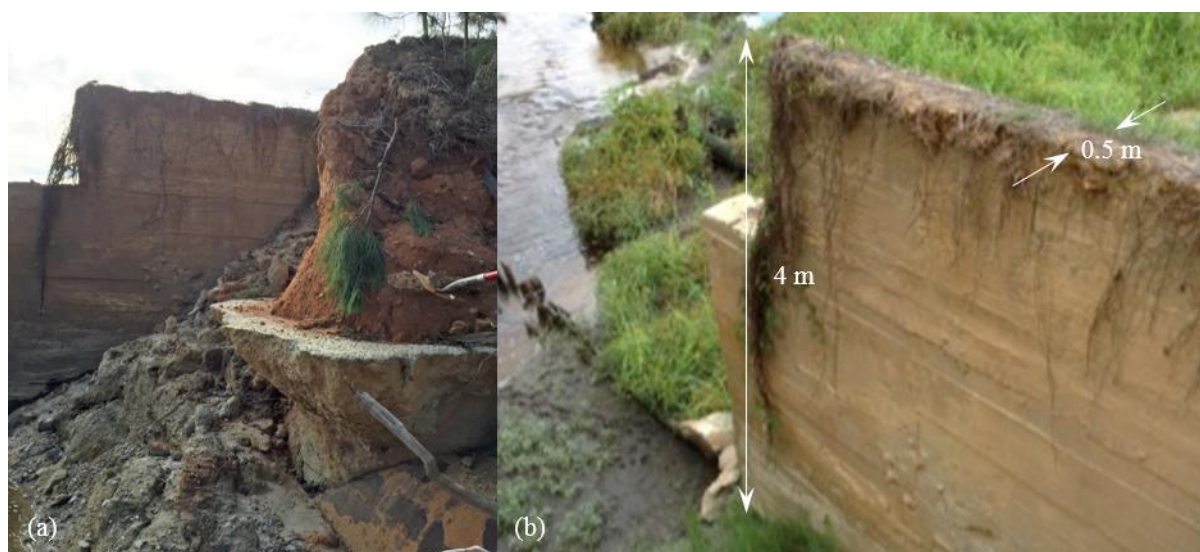
Figure 23. Concrete wall in the upstream section of Dam C, next to the breach zone: a) southwest view from downstream, and b) southeast view from crest of dam.
