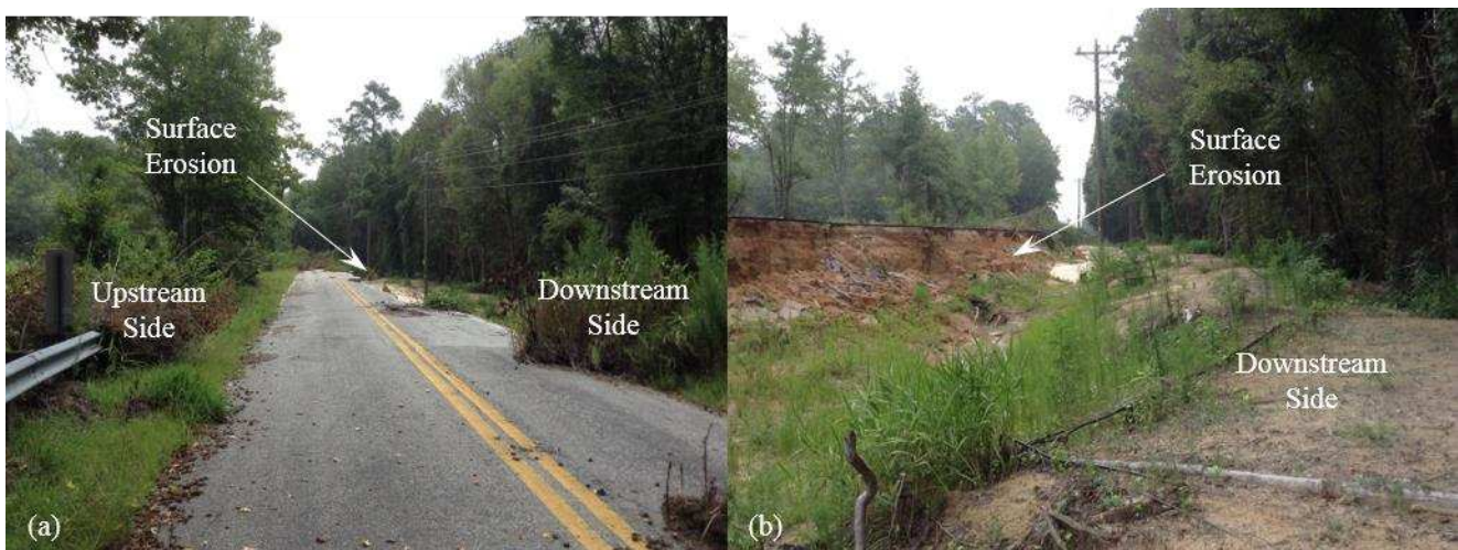
Figure 5. Vegetation on Dam A: (a) vegetation upstream and downstream of the dam (east view from S-40-67), and (b) vegetation and surface erosion on the downstream side of the dam (east view from downstream).
