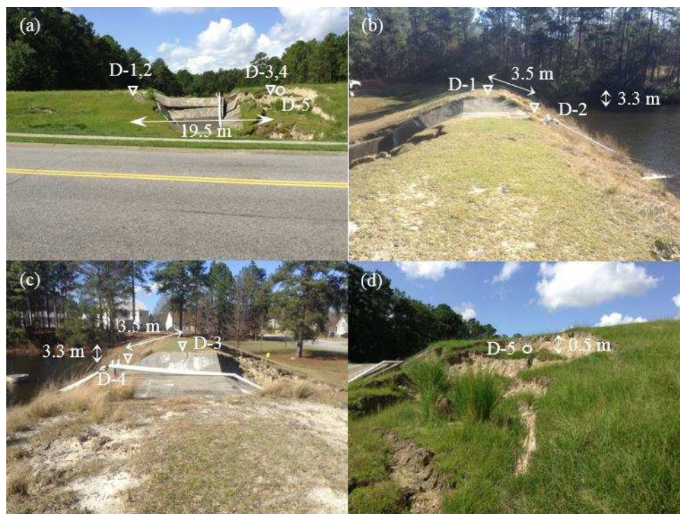
Figure 31. Sampling locations in Dam D: a) southwest view from Legion Drive, b) southeast view from the crest, c) northwest view from the crest, and d) southwest view from downstream side slope near the sliding zone (▽: vertical sample, ○: horizontal sample).
