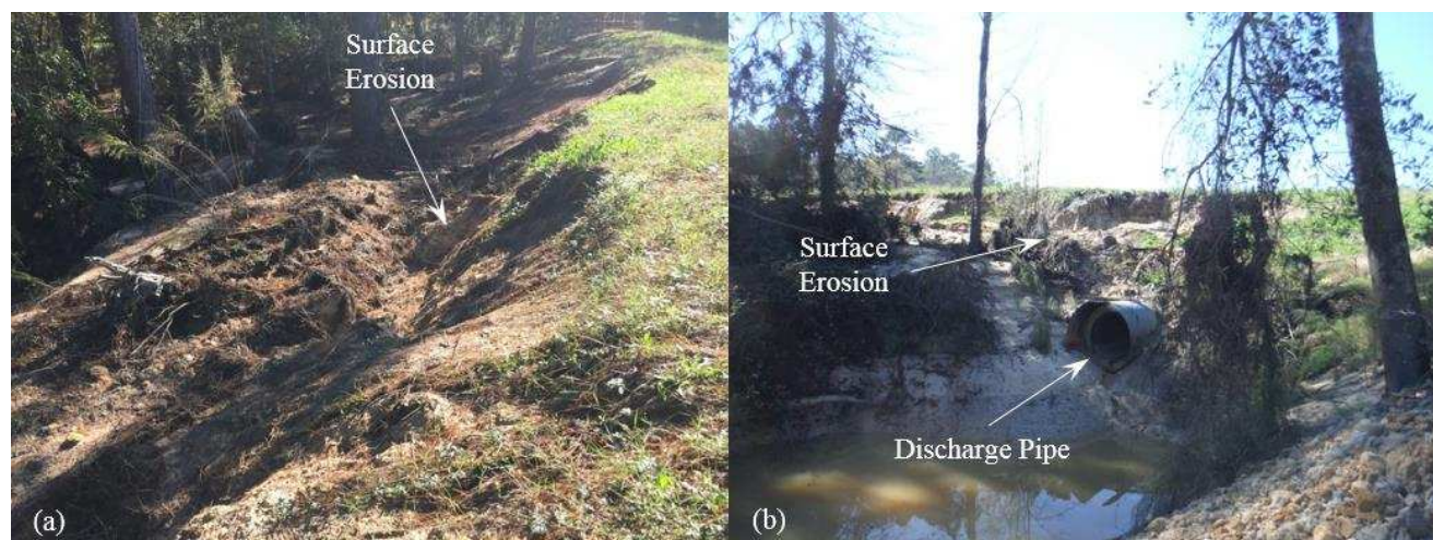
Figure 16. Surface erosion on downstream side slope of Dam B: a) south view from the crest of dam and b) west view from downstream.
