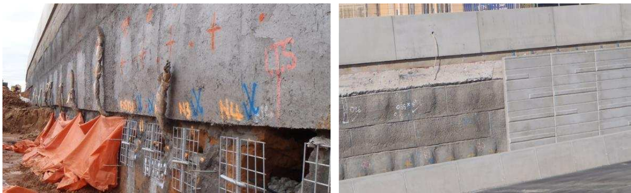
Figure 11. Photographs of wall prepared for shotcreting (left) and shotcreting completed with some facing panels installed (right).
