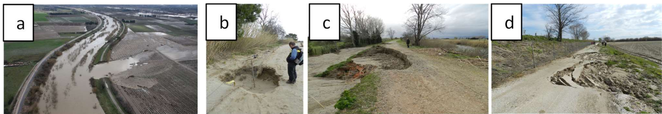
Figure 14. a) The March 2013 breach at the Pia location on the right of the river (photo: DREAL Languedoc-Roussillon), b) A sinkhole close to the breach (photo: Patrice Mériaux, Irstea), c) Damage caused by overflowing (photo: Patrice Mériaux, Irstea), d) Damage to a track on the landward side of the dike caused by under-seepage (photo: Patrice Mériaux, Irstea)
