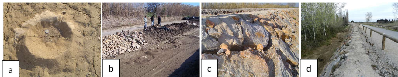
Figure 13. a) Sand boil (photo: Pierre Philippe, CEMAGREF), b) Multiple sand boils close to the maintenance track on the landward side of the dike (photo: Patrice Mériaux, CEMAGREF), c) Damage to the dike itself: cracks on the crest and in the riprap landside revetment (photo: Pierre Philippe, CEMAGREF), d) Damage to the dike itself: crack on the crest; this picture was taken in 2013 but similar damage occurred in 2006 (photo: Patrice Mériaux, Irstea).
