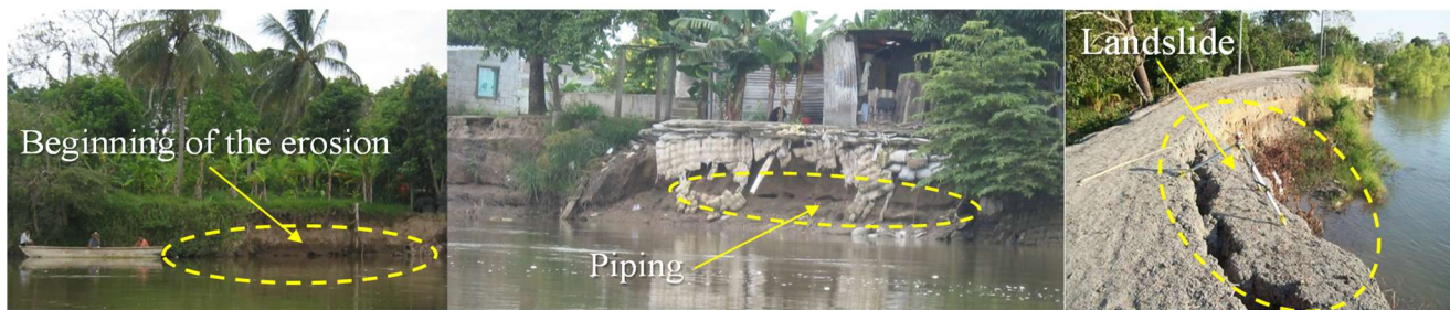
Figure 4. Evidence of instability in river banks and dikes induced by rapid drawdown in Villahermosa.
