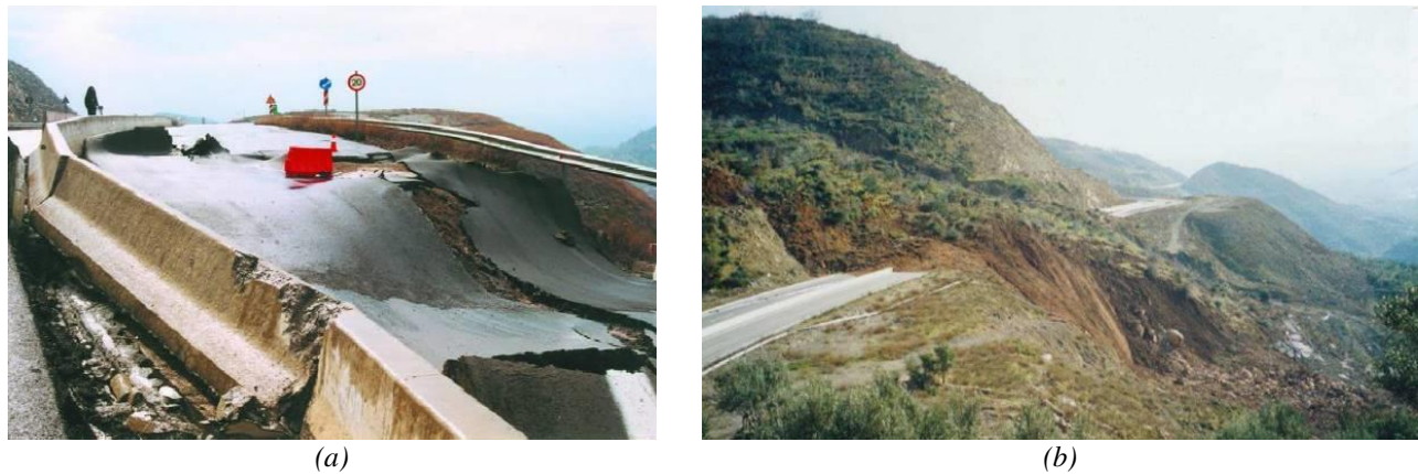
Figure 1. The Tsakona landslide (February 2003) (EMEK S.A (2015)) (a) large settlements on the road pavement (b) massive soil movement (Fikiris et al. (2001)).
