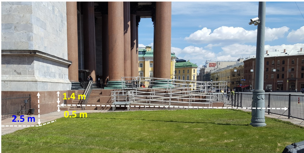
Figure 15. Settlement measurements at the southwest corner.
