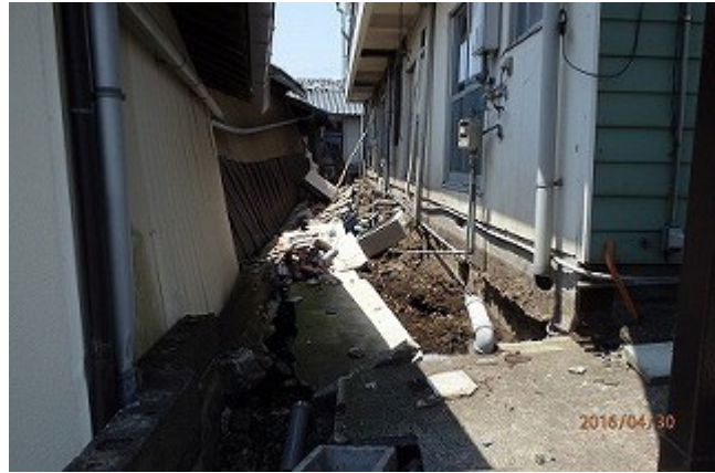
Figure 17. Ground displacement-induced damage to a residential house (Site 9 in Fig. 12) ( 32^{\circ} 47'14.48''N , 130^{\circ} 48'41.06''E ).
