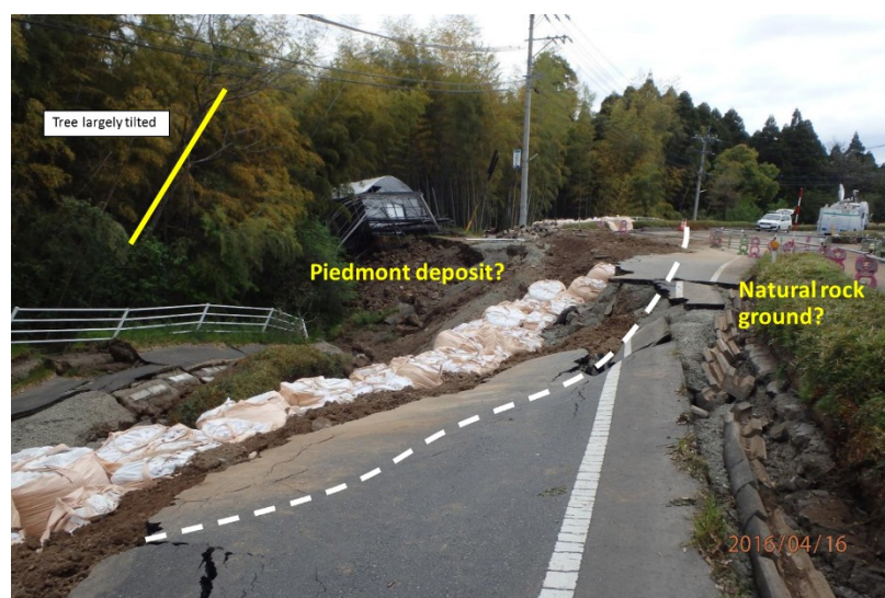
Figure 18. Damage to Route 443 in Mashiki Town (Site 10 in Figs. 12 and 14) ( 32^{\circ} 47'29.71''N , 130^{\circ} 49'17.58''E ).
