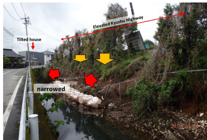
Figure 10. Damage to Kyushu Highway embankment (Site 6 in Figs. 3 and 7) ( 32^{\circ} 46'46.80''N , 130^{\circ} 47'39.40''E ).
