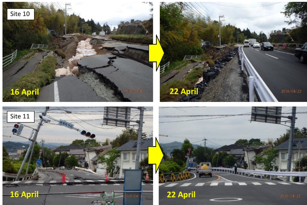
Figure 19. Damages to Route 443 and their restoration for (a) site 10 and (b) site 11 (c.f. Figs. 12 and 14) (Site 10: 32^{\circ}47'29.71''N , 130^{\circ}49'17.58''E , Site 11: 32^{\circ}47'24.33''N , 130^{\circ}49'15.82''E ).
