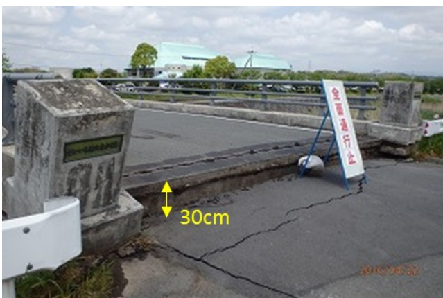
Figure 8. A large gap at bridge girder due to settlement of embankment (Site 4 in Fig. 3) ( 32^{\circ} 47'2.15''N , 130^{\circ} 49'17.70''E ).
