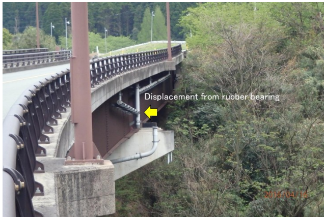
Figure 24. The girder of Ohkirihata Bridge moved about 1-1.5m (Site 14 in Fig. 12) ( 32^{\circ} 50'32.63''N , 130^{\circ} 55'43.10''E ).
