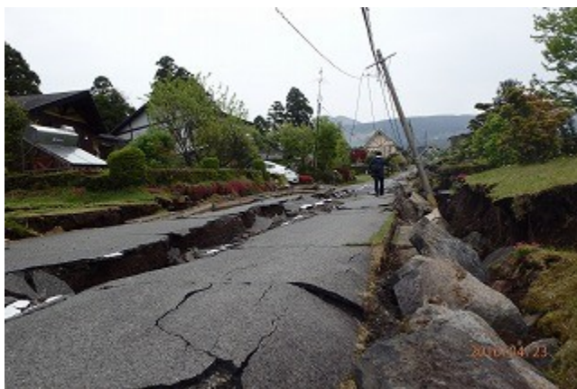
Figure 32. Damage to the road in residential area developed by filling (Site 21 in Fig. 26) ( 32^{\circ} 52'43.89''N , 130^{\circ} 59'58.89''E ).
