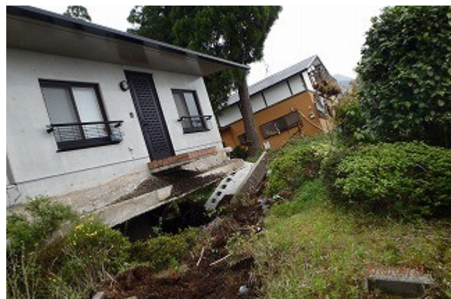
Figure 33. Damage to the house in residential area developed by filling (Site 21 in Fig. 26) ( 32^{\circ} 52'45.06''N , 131^{\circ} 00'1.44''E ).
