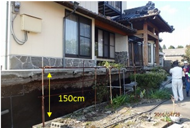
Figure 36. Ground depression-induced damage to the residential house (Site 23 in Fig. 26) ( 32^{\circ} 57'23.84''N , 131^{\circ} 2'12.31''E ).
