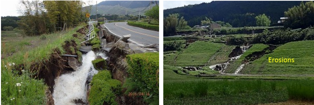
Figure 21. Damage to road embankment along prefectural road No. 28 (site 13 in Fig. 12) ( 32^{\circ}50'36.63''N , 130^{\circ}55'24.48''E ).
