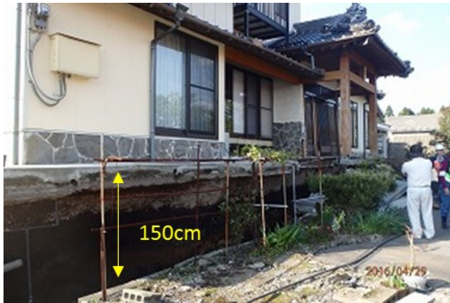
Figure 36. Ground depression-induced damage to the residential house (Site 23 in Fig. 26) ( 32^{\circ} 57'23.84''N , 131^{\circ} 2'12.31''E ).
