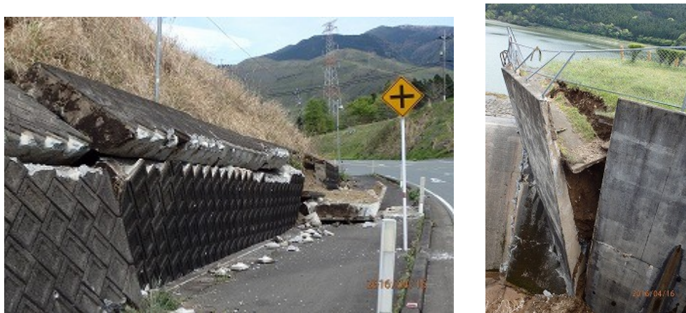
Figure 20. Damage to retaining wall and spillway retaining wall (site 12 in Fig. 12) ( 32^{\circ}50'29.22''N , 130^{\circ}55'55.83''E ).
