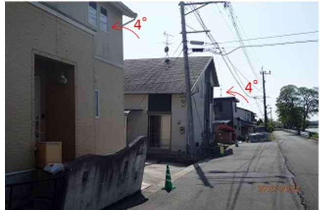
Figure 5. Liquefaction-induced damage to residential houses in Majima district (Site 2 in Fig. 3) ( 32^{\circ} 45'52.69''N , 130^{\circ} 46'7.49''E ).
