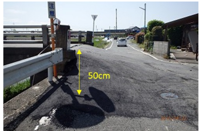
Figure 9. Temporary restoration work (filled slope) for settlement of levee (Site 5 in Figs. 3 and 7) ( 32^{\circ} 46'44.47''N , 130^{\circ} 47'45.43''E ).
