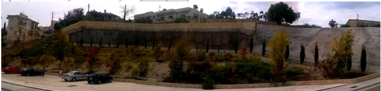
Figure 22. The landslide back scarp area after its stabilization by installing a permanent anchored wall.
