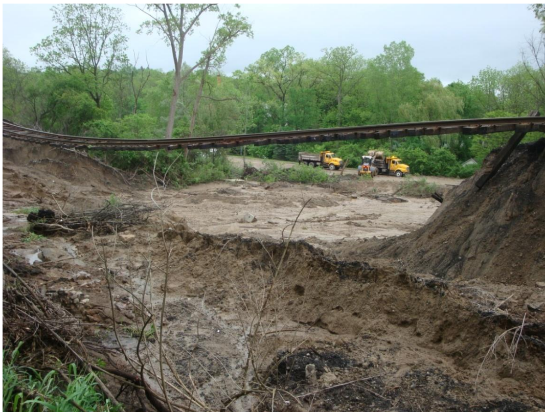
Figure 7. View of the failure along, and perpendicular to, the railroad embankment axis.
