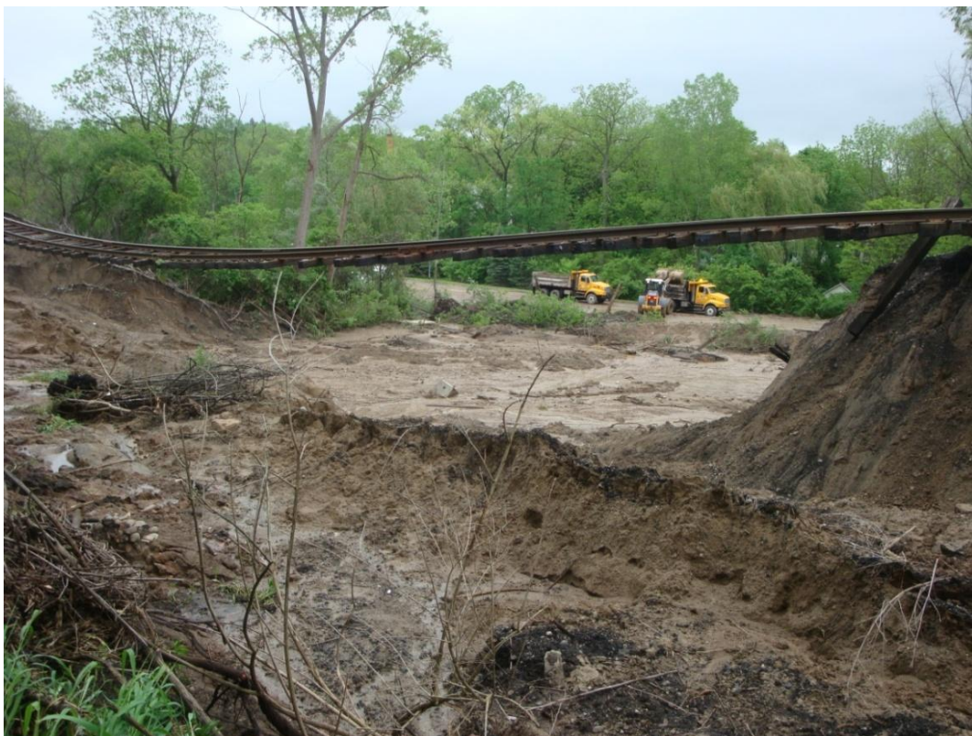
Figure 7. View of the failure along, and perpendicular to, the railroad embankment axis.
