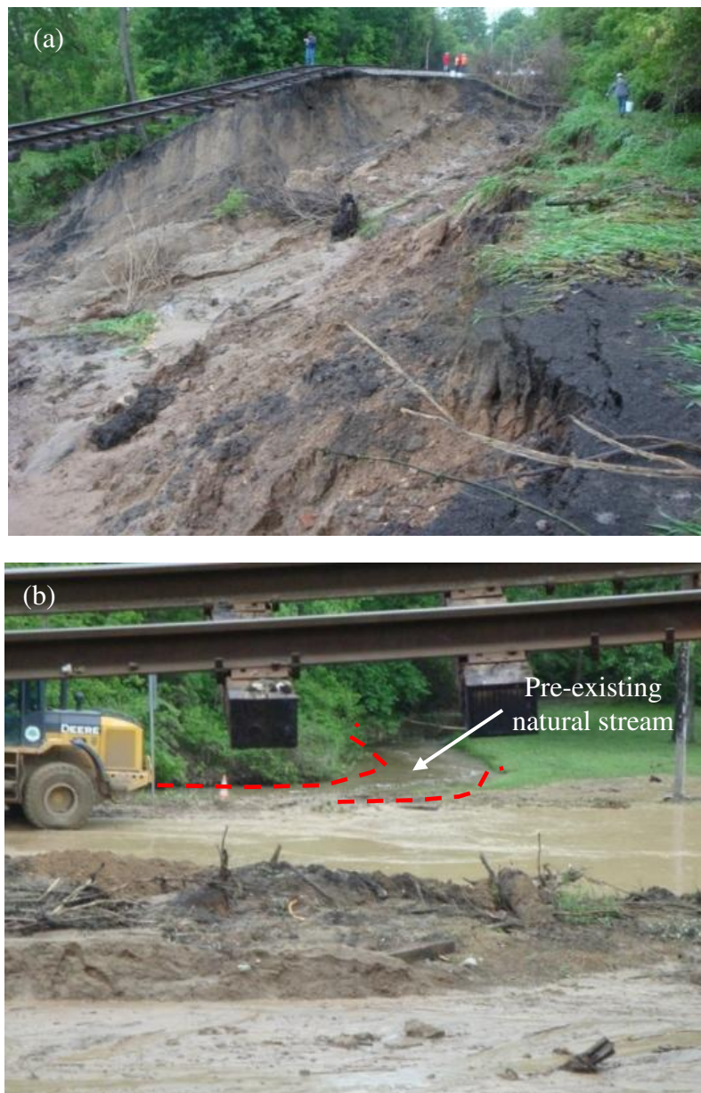
Figure 10. View of the failure from the crest of the failure surface where (a) the left-in-place embankment is shown; (b) the mass of soil with large amount of water is shown at the toe of the failure reaching the pre-existing natural stream.
