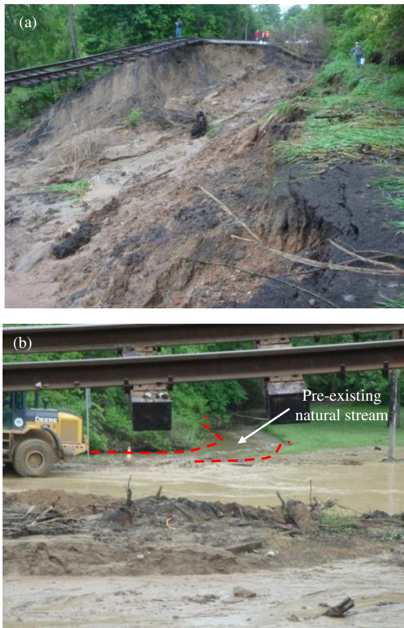
Figure 10. View of the failure from the crest of the failure surface where (a) the left-in-place embankment is shown; (b) the mass of soil with large amount of water is shown at the toe of the failure reaching the pre-existing natural stream.
