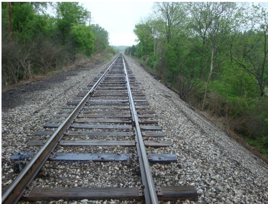
Figure 3. View of intact portion of the embankment immediately to the East of the failure area. One can see that the uphill part of the embankment (left) is supported by natural ground that is at a much higher elevation than the downhill part of the embankment (right).
