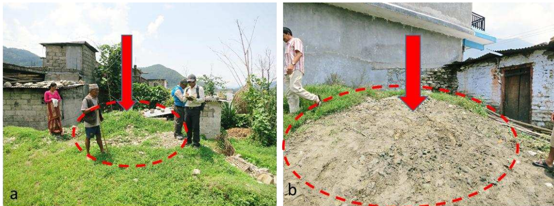
Figure 6. Typical effects of sinkhole formation on residential properties observed on June 2014 included the collapsed of (a) a cowshed and (b) a masonry kitchen.
