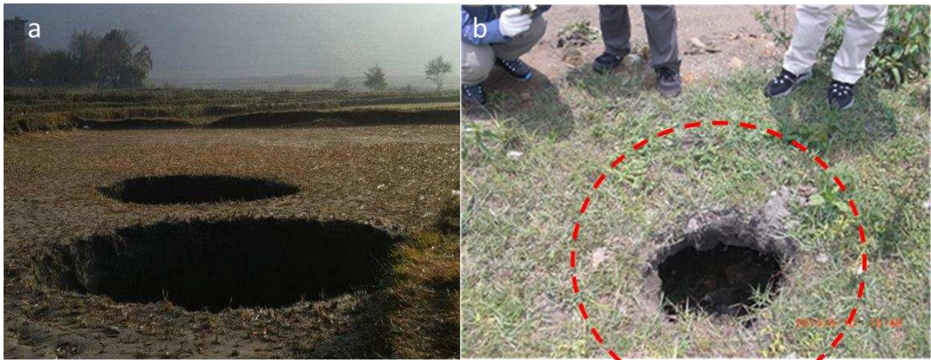
Figure 5. (a) Typical sinkholes formed in November 2013 (Photo Courtesy: Keshab Sharma); and (b) a sinkhole formed in June 2014 (photo point 2).
