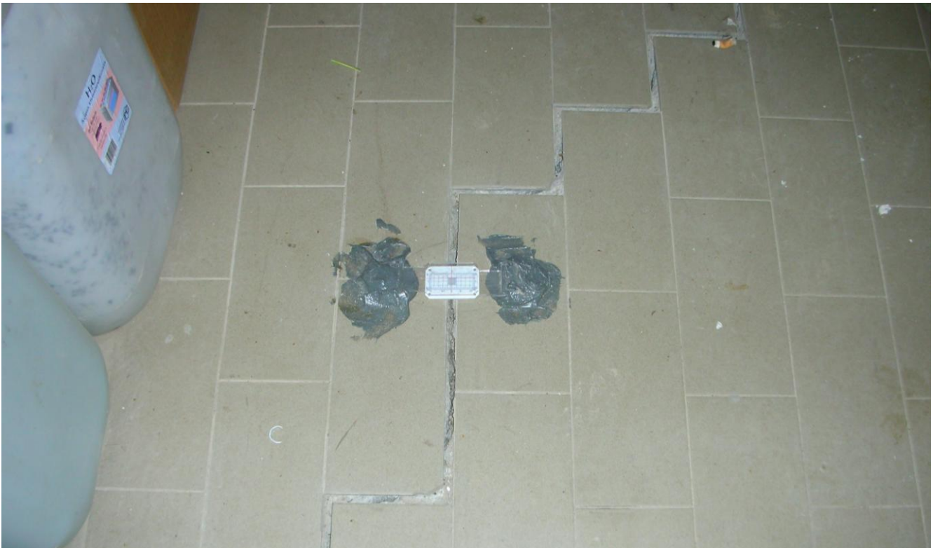
Figure 3. Floor damage inside the warehouse.
