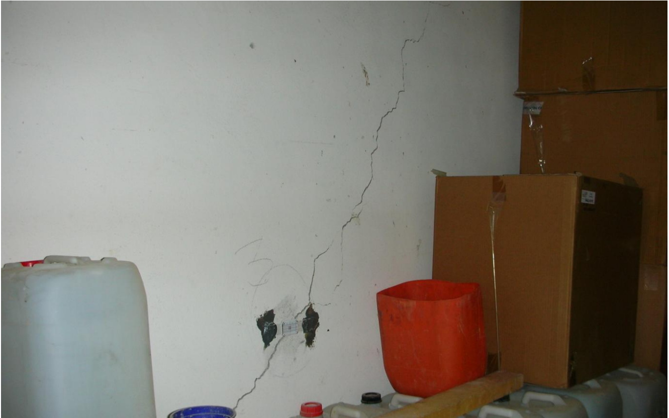
Figure 2. Wall damage inside the warehouse.
