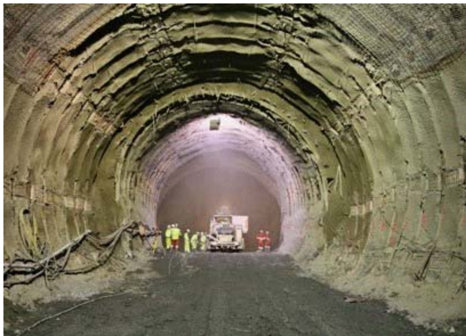
Figure 9. Photograph of the tunnel with the DSM support system installed. The HiDCon elements inserted in the shotcrete lining are well visible.
