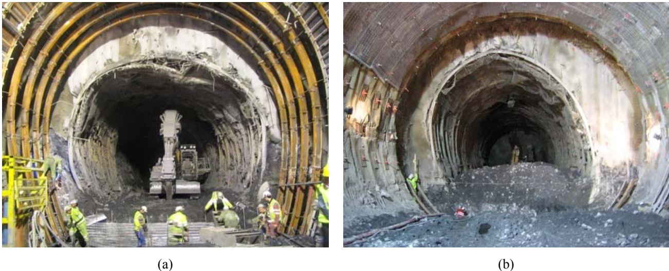
Figure 1. Squeezing rock reduces the tunnel cross section in the Saint Martin La Porte access adit (Lyon-Turin Base Tunnel). The photographs show re-mining works needed in order to cope with the difficult conditions encountered.
