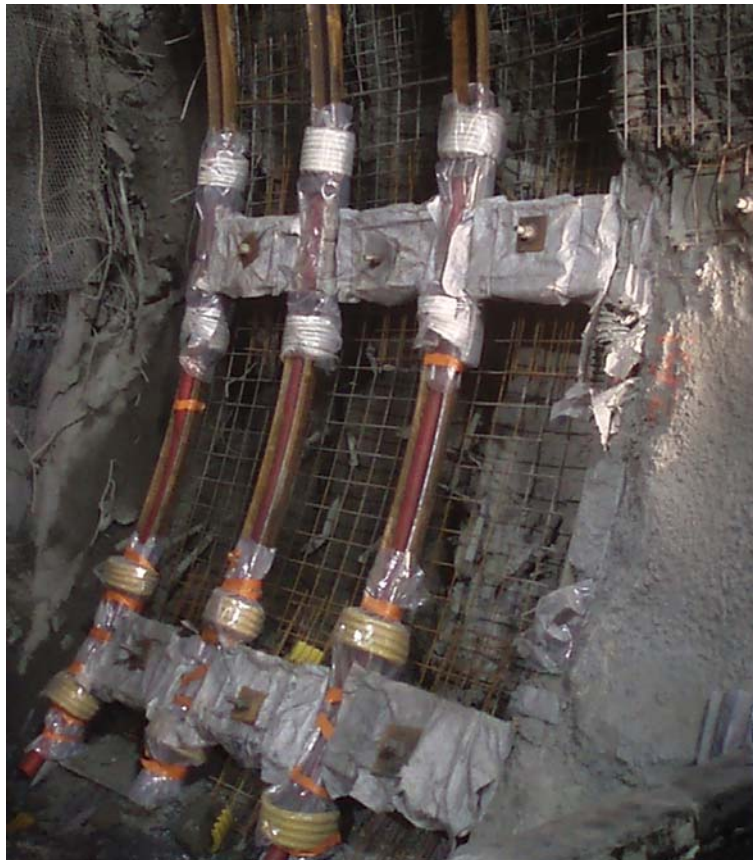
Figure 8. Detail of the installation of the TH steel sets and HiDCon elements.
