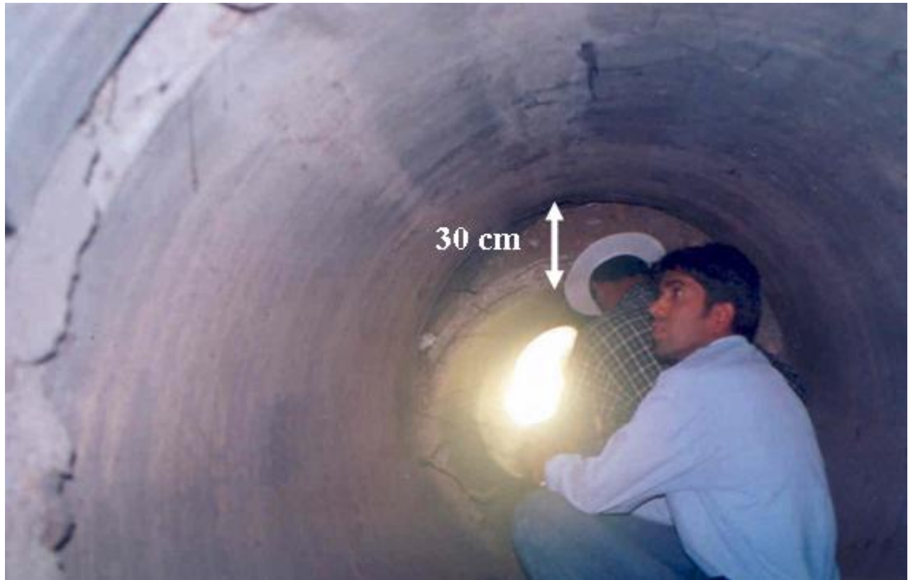
Figure 11. Dislodged pipe culvert.
