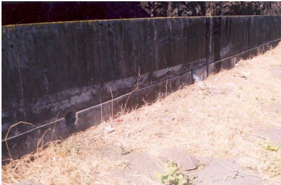
Figure 15. Drainage holes left open on embankment surface.
