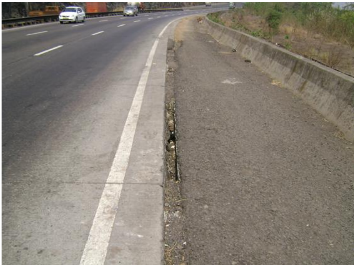
Figure 14. Crack between rigid and bituminous pavement.
