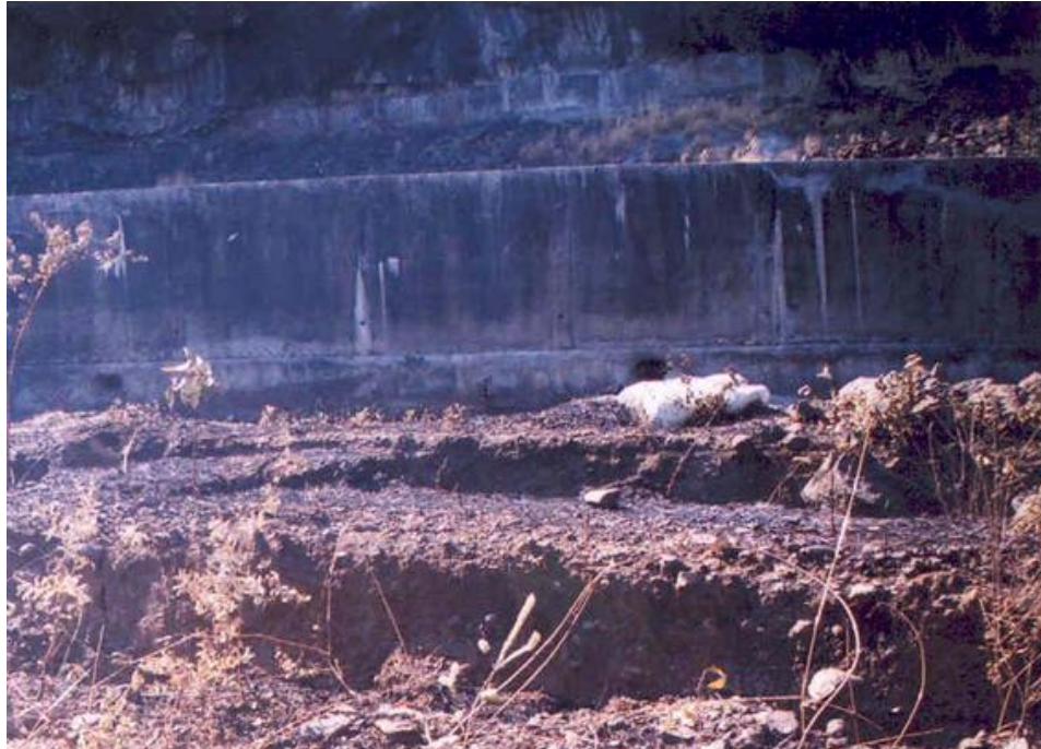
Figure 17. Subsidence of the embankment.
