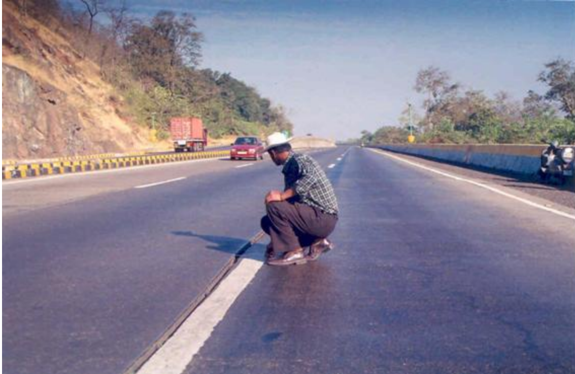
Figure 13. Dislodged rigid pavement.
