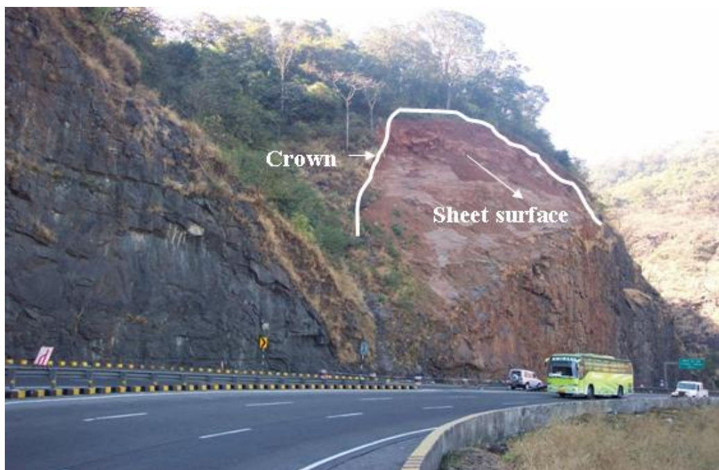
Figure 2. General view of rockfall and debris.
