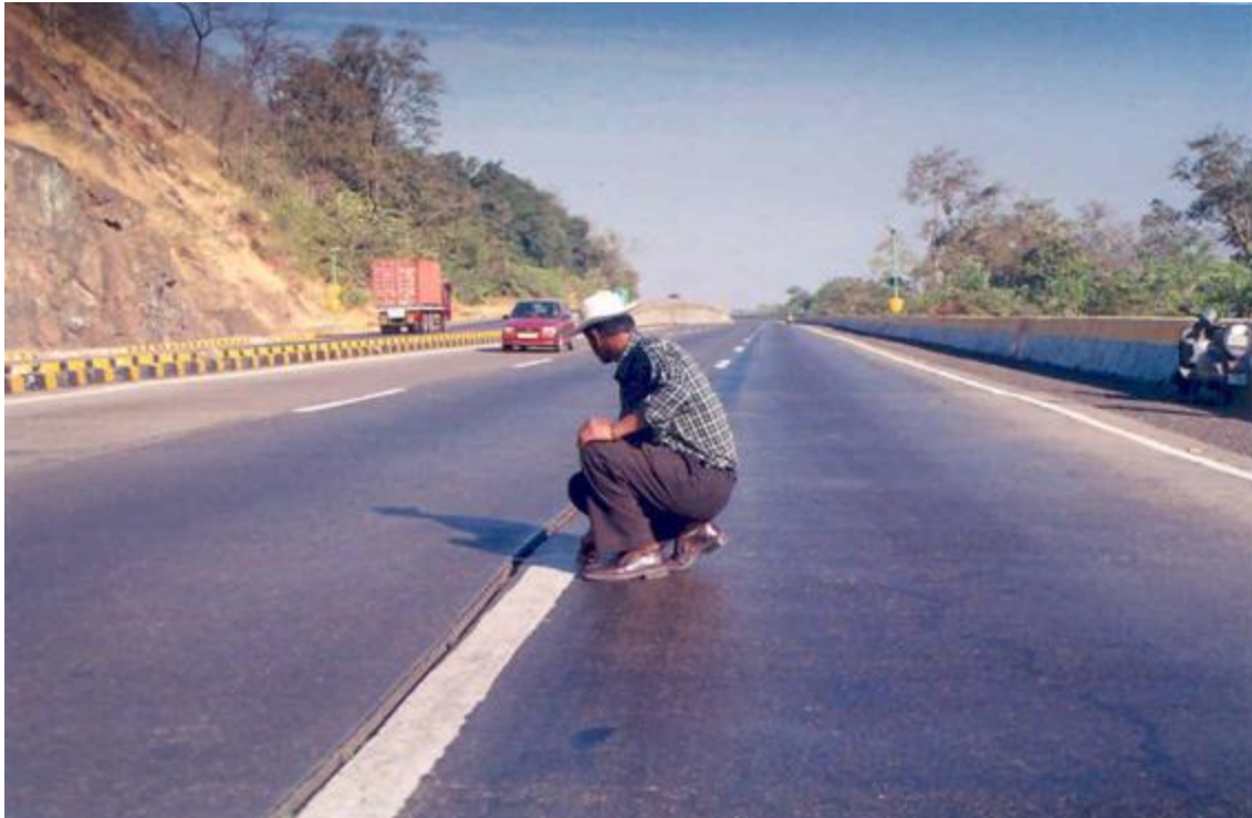
Figure 13. Dislodged rigid pavement.
