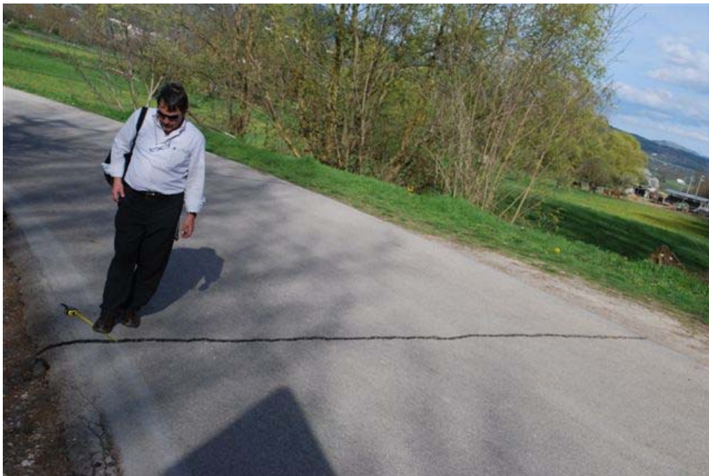
Figure 141. Characteristic crack developed in bridge approach road directly south of Onna, at distances of 15 m to 160 m from the Aterno River (42.324N, 13.478E).
