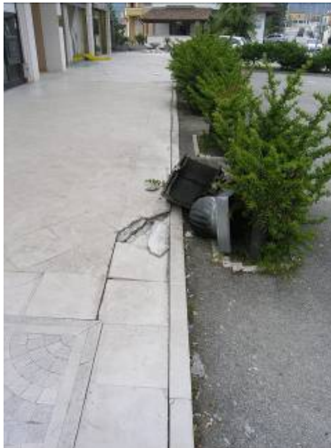
Figure 33. Separation cracks at sidewalk on front of building (42.359335°N, 13.468954°E).
