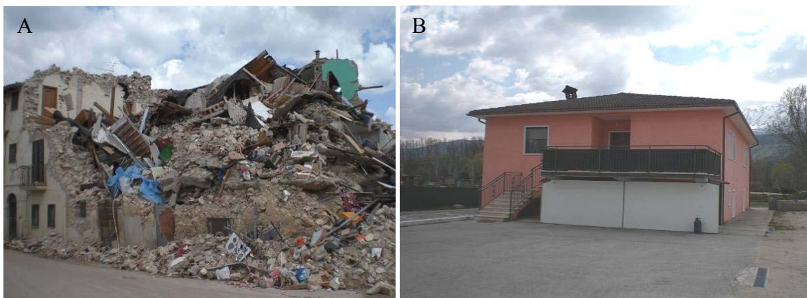
Figure 67. Onna. (A) D5 damage level on masonry building structures, (B) D0 damage on a RC building (except for the tilting of the chimney).
