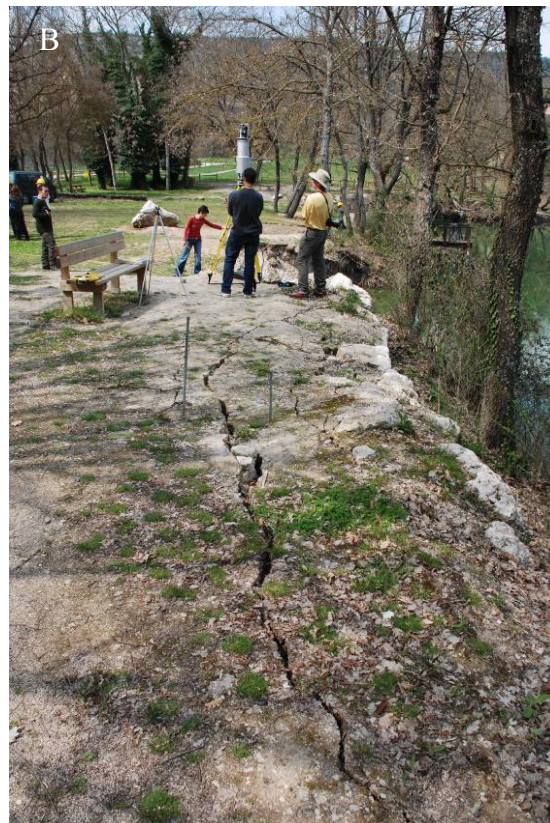
Figure 162. Ground cracks at the southwest corner of Lake Sinizzo (location WP 18) as observed on (B) 15 April 2009.
