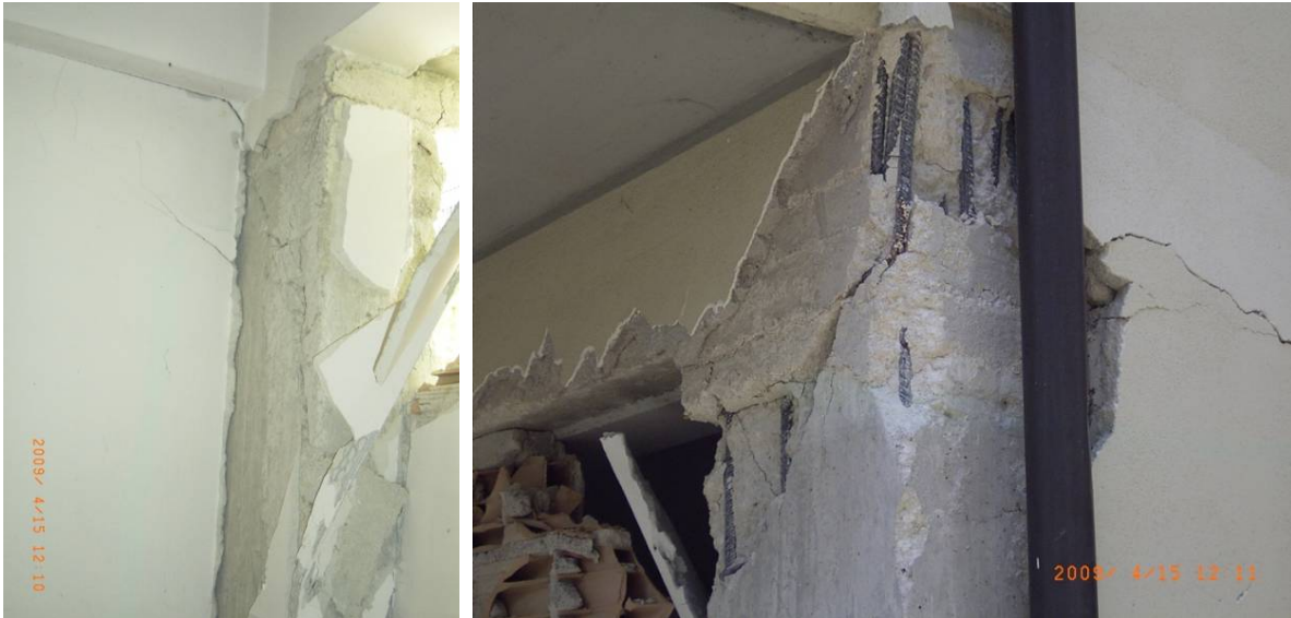
Figure 105. Example of D3 damage in the building at waypoint GB-88-1.
