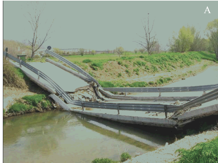
Figure 68. Onna. (A) Collapse (D5).
