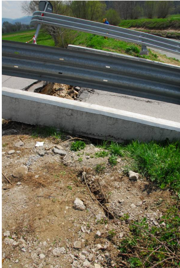
Figure 148. Ground cracking in levee directly beneath western abutment along northern side of Aterno River (42.325N, 13.463E).
