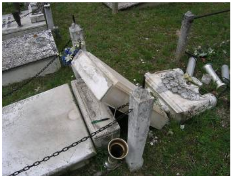
Figure 49. Grave markers breakage.
