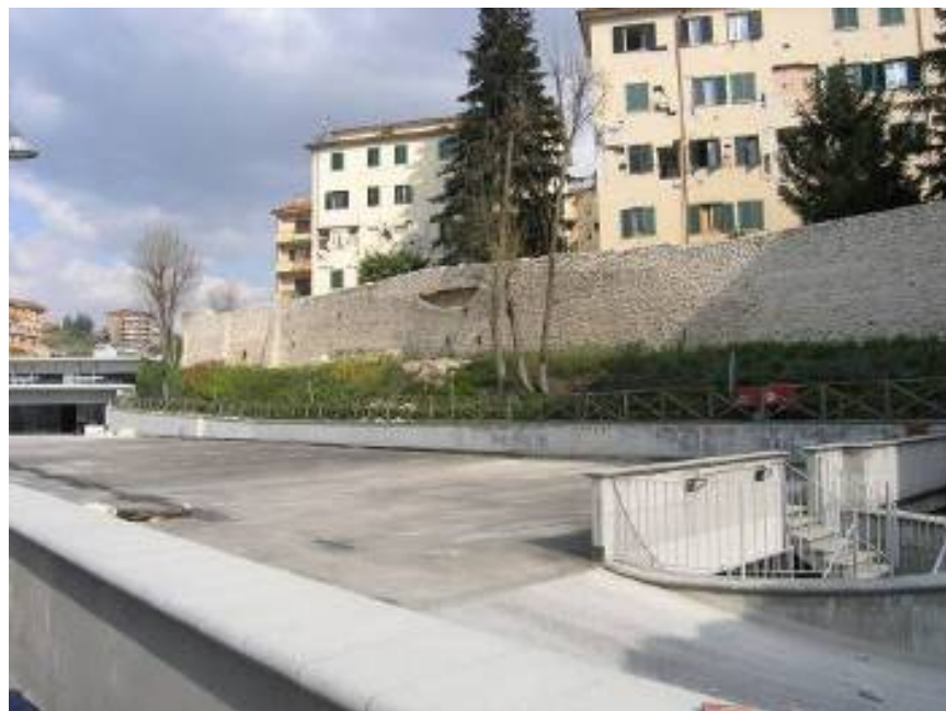
Figure 188. Damaged wall at downtown L'Aquila ( 42.356056^{\circ}\text{N} , 13.389524^{\circ}\text{E} ).
