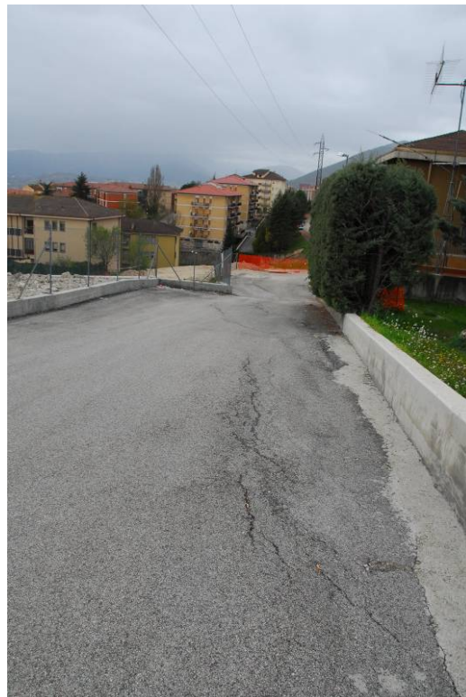
Figure 154. Cracks in the overlying asphaltic surfaces and a narrow settlement trend along the sidewall of the cut-and-cover structure (42.358N 13.415E).
