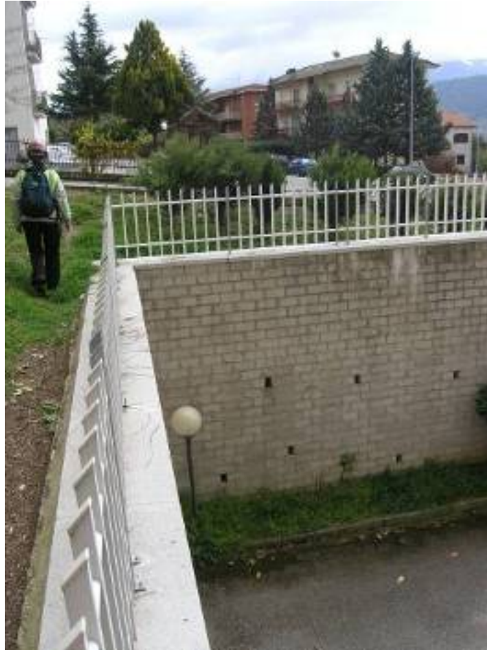
Figure 187. Undamaged wall at the severely shaken Pettino area ( 42.373050^{\circ}\text{N} , 13.366106^{\circ}\text{E} ).
