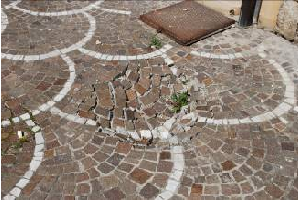
Figure 30. Local settlement close to piping system (42.359335°N, 13.468954°E).
