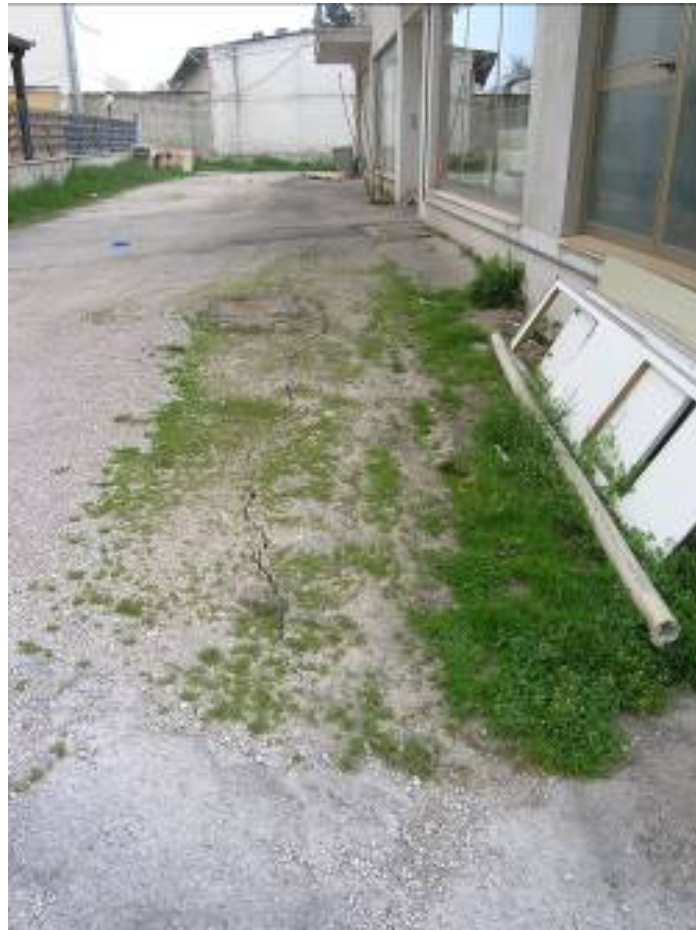
Figure 31. Ground fissures at the side of the building (42.359817°N, 13.468649°E).
