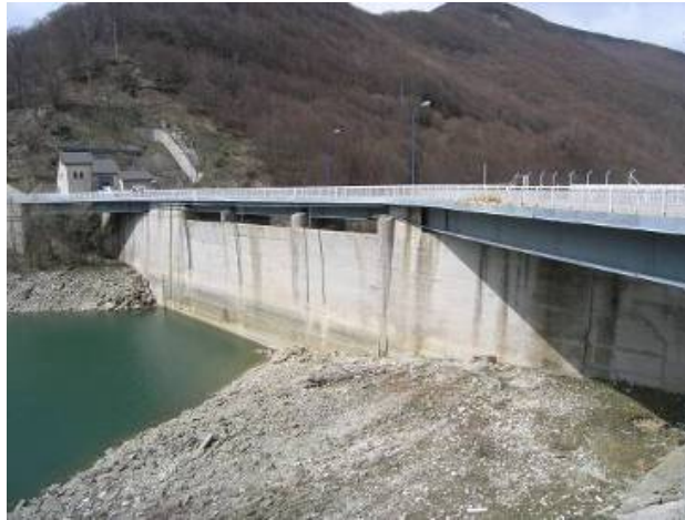
Figure 179. Upstream face of Rio Fucino dam. Note the lowering of water level (42.535047°N, 13.410323°E).
