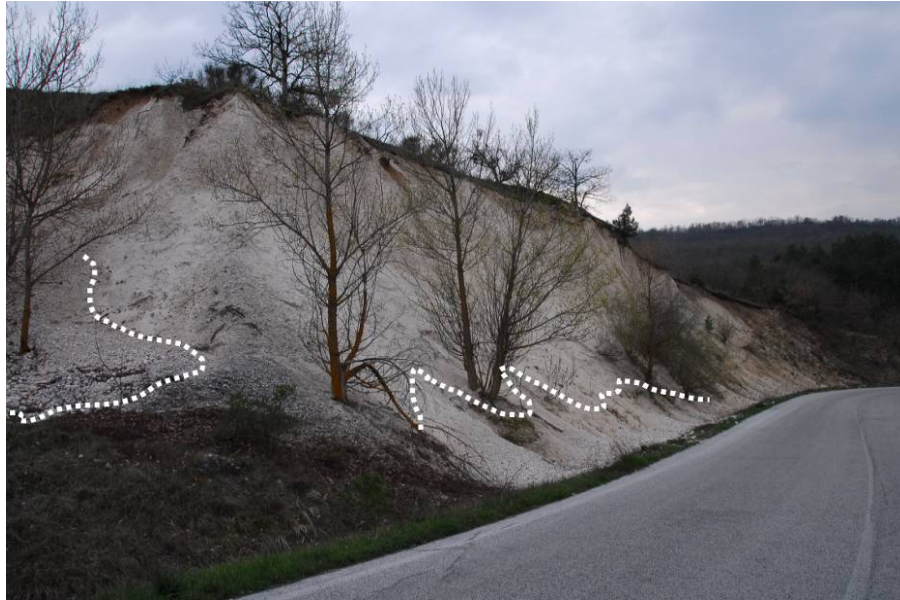
Figure 121. Minor ravelling of weakly cemented sand and gravel; dashed lines indicate the extent of freshly deposited talus along the base of road cut (Via Opi N42.261, E13.581).
