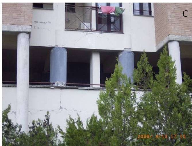
Figure 110. Damage on the structures in the cluster in zone (d). (C) Waypoint GB-26-1 (D2).
