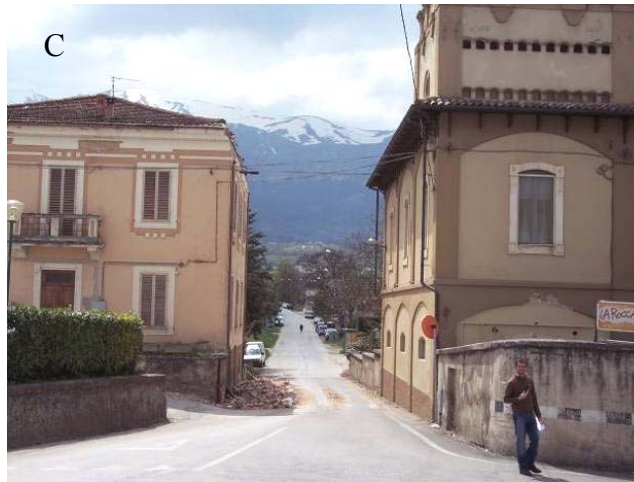
Figure 70. Monticchio. (C) D1 damage (fall of the cornice) on a masonry building.
