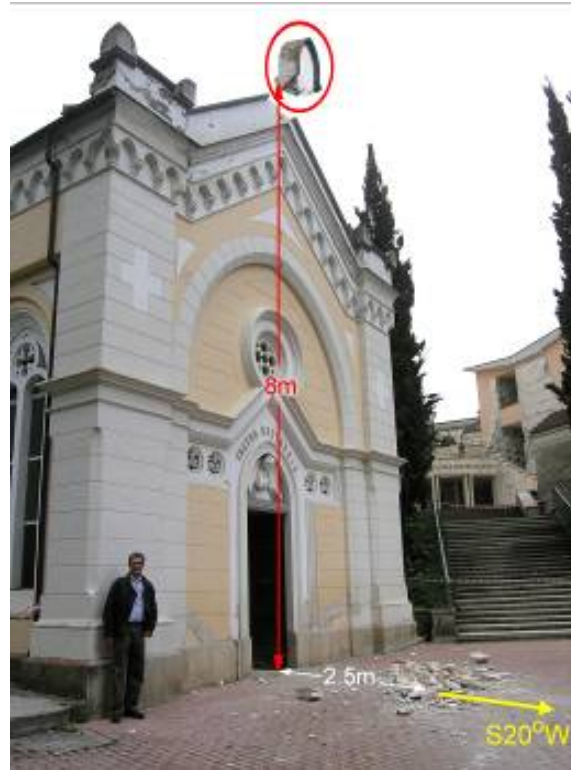
Figure 53. Fall of facade object at mortuary building.
