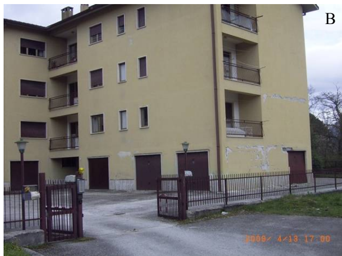
Figure 110. Damage on the structures in the cluster in zone (d). (B) Waypoint GB-25-1 (D2).
