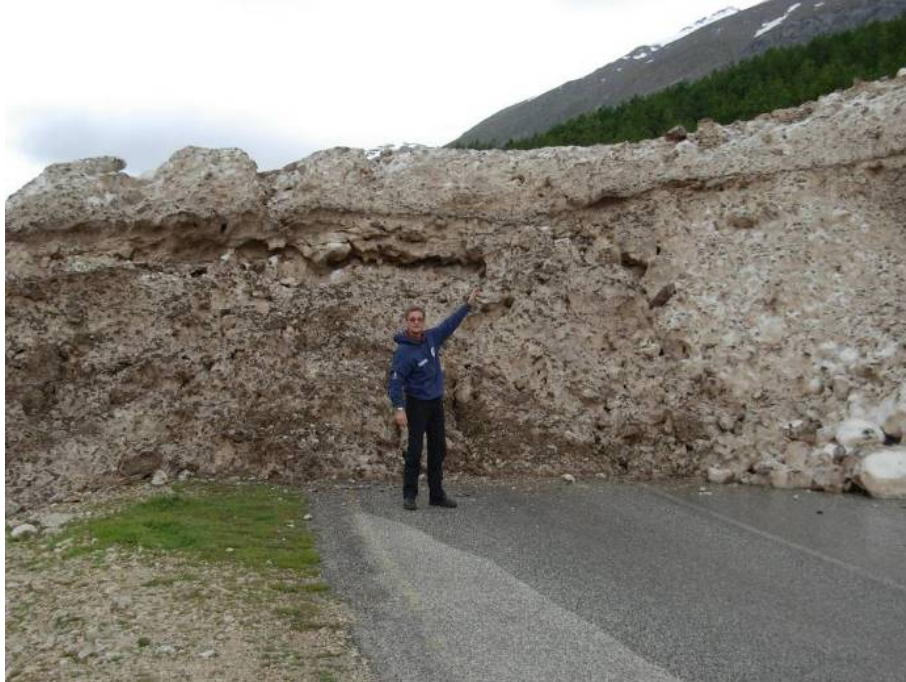
Figure 137. Debris flow body invading the SP86. (Courtesy of Dr. Roberta Giuliani, DPC-SISM) (42.4368N, 13.5796E).
