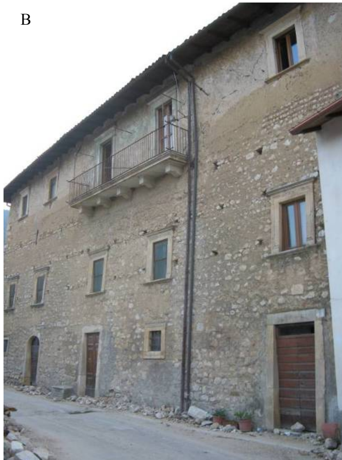
Figure 88. Villa S. Angel. (B) Reinforced masonry in the historic center with minor cracks in the highest story (D2).
