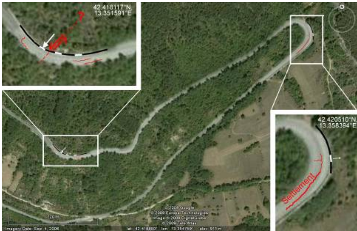
Figure 191. Locations of observed pavement cracking and associated retaining wall failures.
