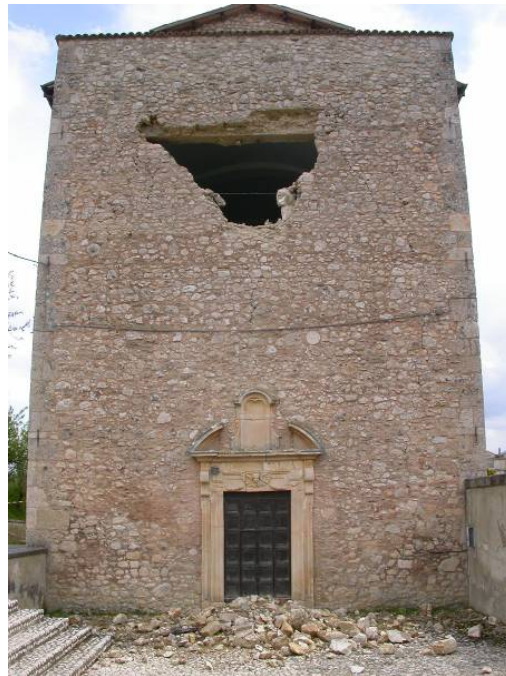
Figure 81. S. Eusanio Forconese: partial collapse of the masonry church (D4).
