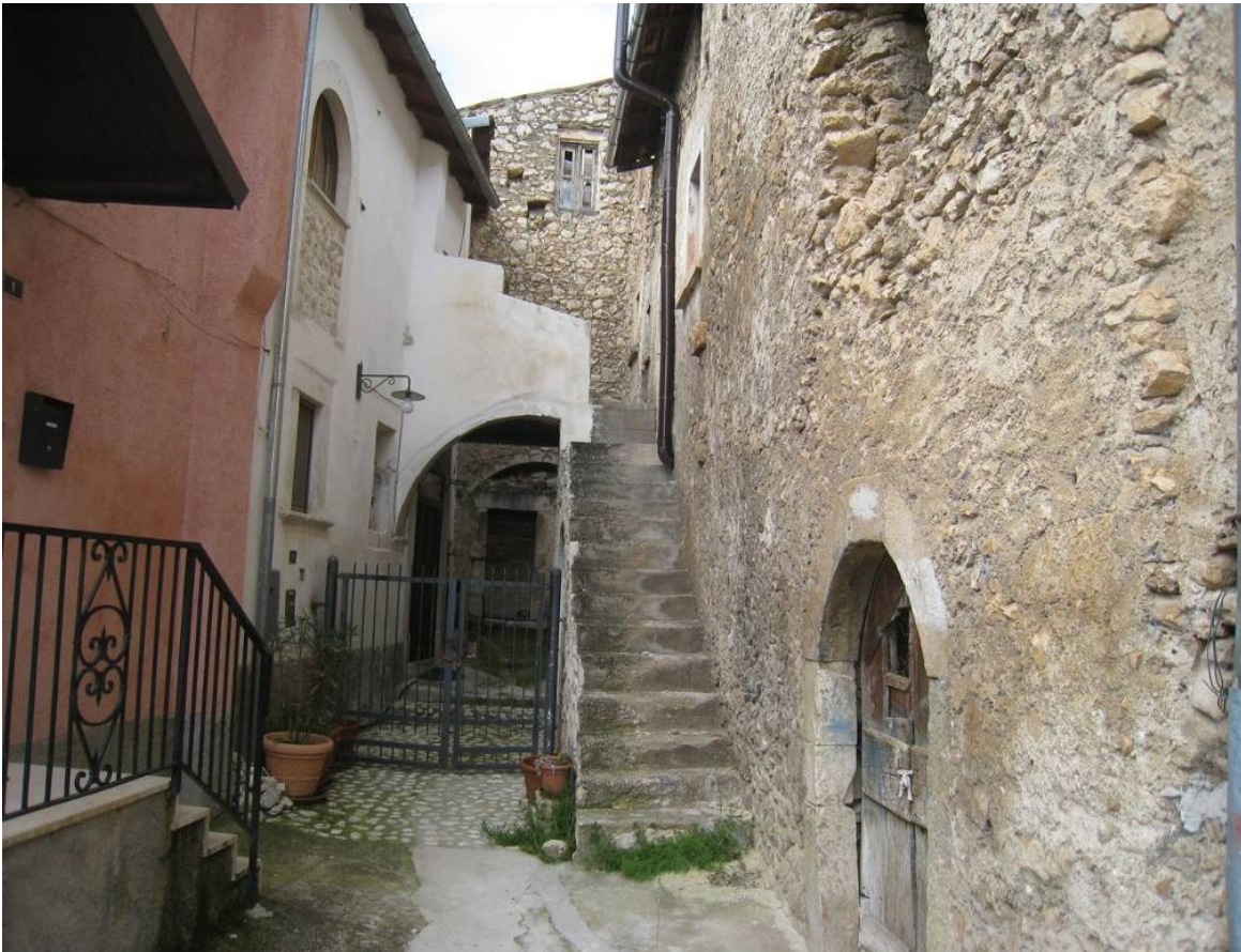
Figure 62. Typical unreinforced masonry structures in the village of San Pio delle Camere suffered no damage (D0), or slight cracking (D1). Structures in this village are similar to those in Castelnuovo. San Pio delle Camere is built on limestone bedrock.
