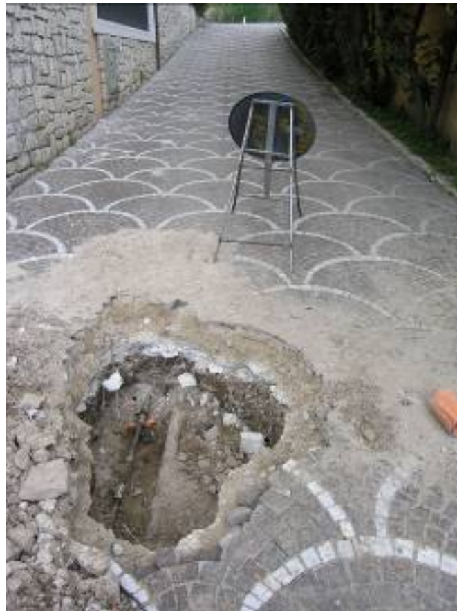
Figure 29. Failure of water pipe. (42.359335°N, 13.468954°E).
