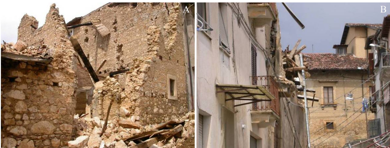
Figure 80. S. Eusanio Forconese. (A) Collapse of old masonry building (D5), (B) Partial collapse of masonry building (D4).
