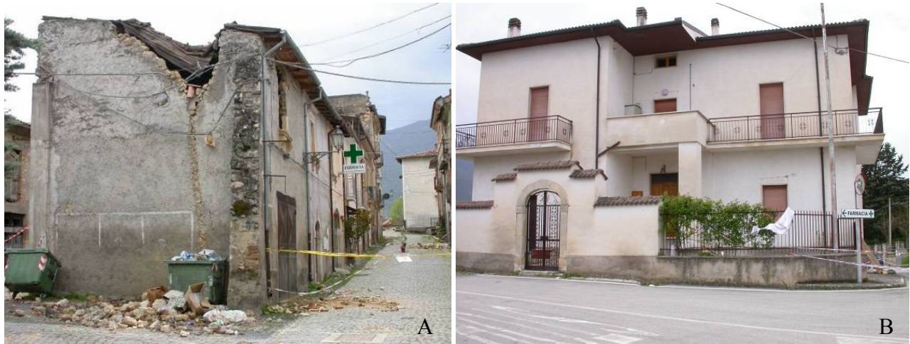
Figure 79. S. Eusanio Forconese village. (A) Partial collapse of masonry building (D4), (B) Slight damage to a RC building nearby (D1).
