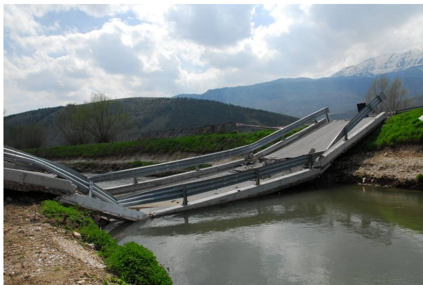
Figure 145. Bridge collapse along the Aterno River, approximately 450 m north of Monticchio (42.325N, 13.463E).
