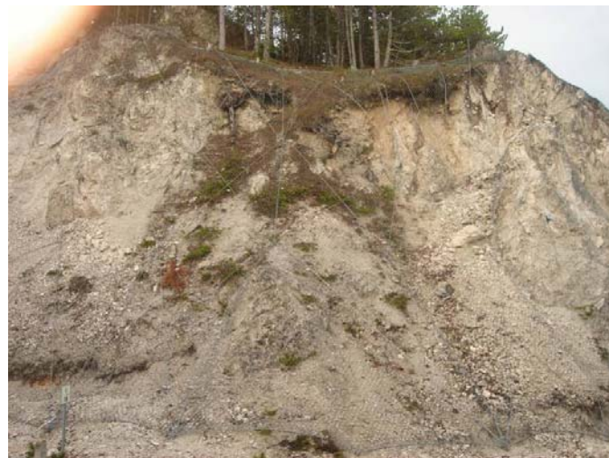
Figure 131. Ravelling in pervasively fractured/cataclastic limestones on a road cut retained by steel-net protections on SS80 at km 18.2: (DC-18-1) (42.4281N, 13.3460E).
