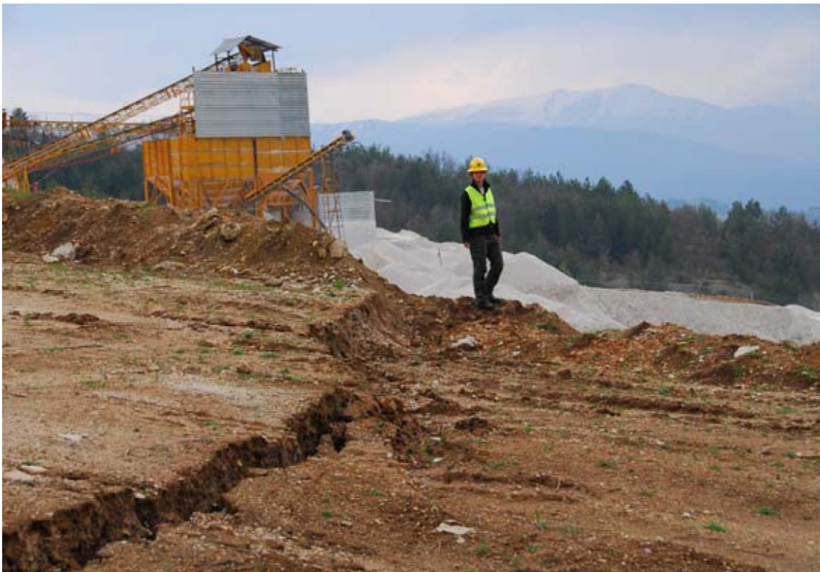
Figure 149. Shear failure developed in fill material, with vertical displacement increasing to approximately 40 cm at free slope face (42.435N, 13.330E).
