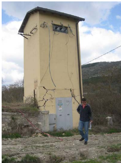
Figure 57. Heavily damaged seismometer station box (not in use at the time of the earthquake, no recording) on the northeast valley beneath the town of Castelnuovo. (42.2982°, 13.6295°).
