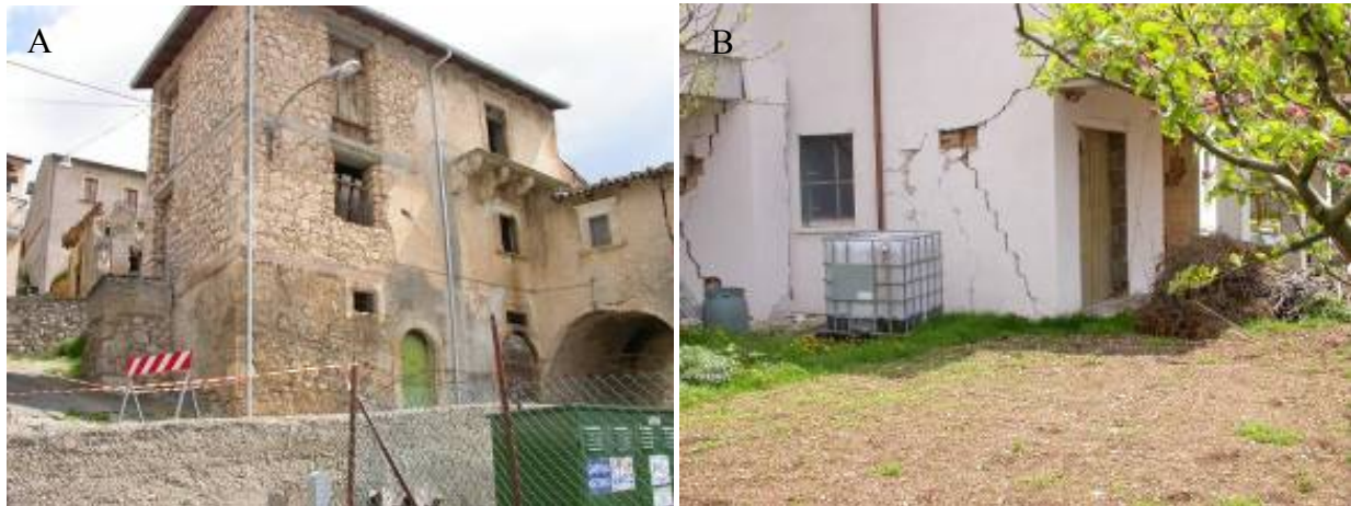
Figure 96. Barisciano. (A) Collapse (D5) of an old masonry building in background, (B) Damages (D1/D2) to RC buildings.
