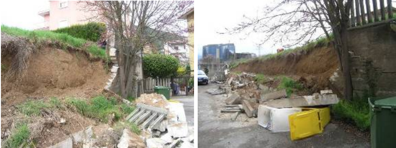
Figure 193. Toppling of masonry retaining wall at the outskirts of L'Aquila (42.366803°N, 13.376561°E).
