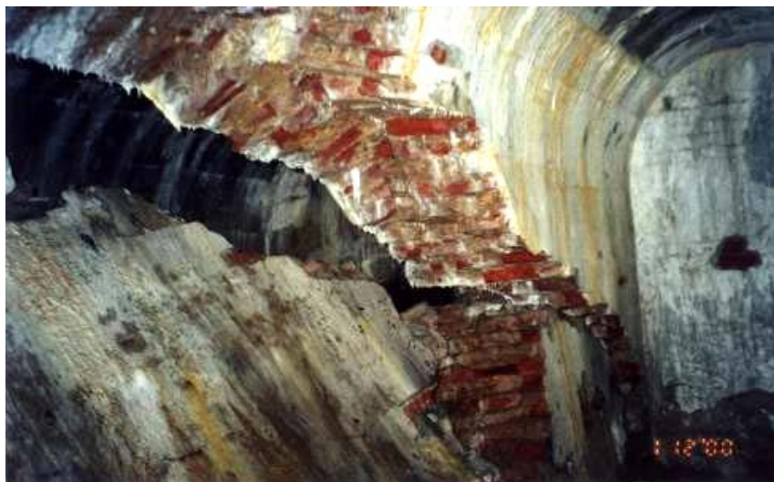
Figure 10. Collapsing cellar wall behind east loggias.
