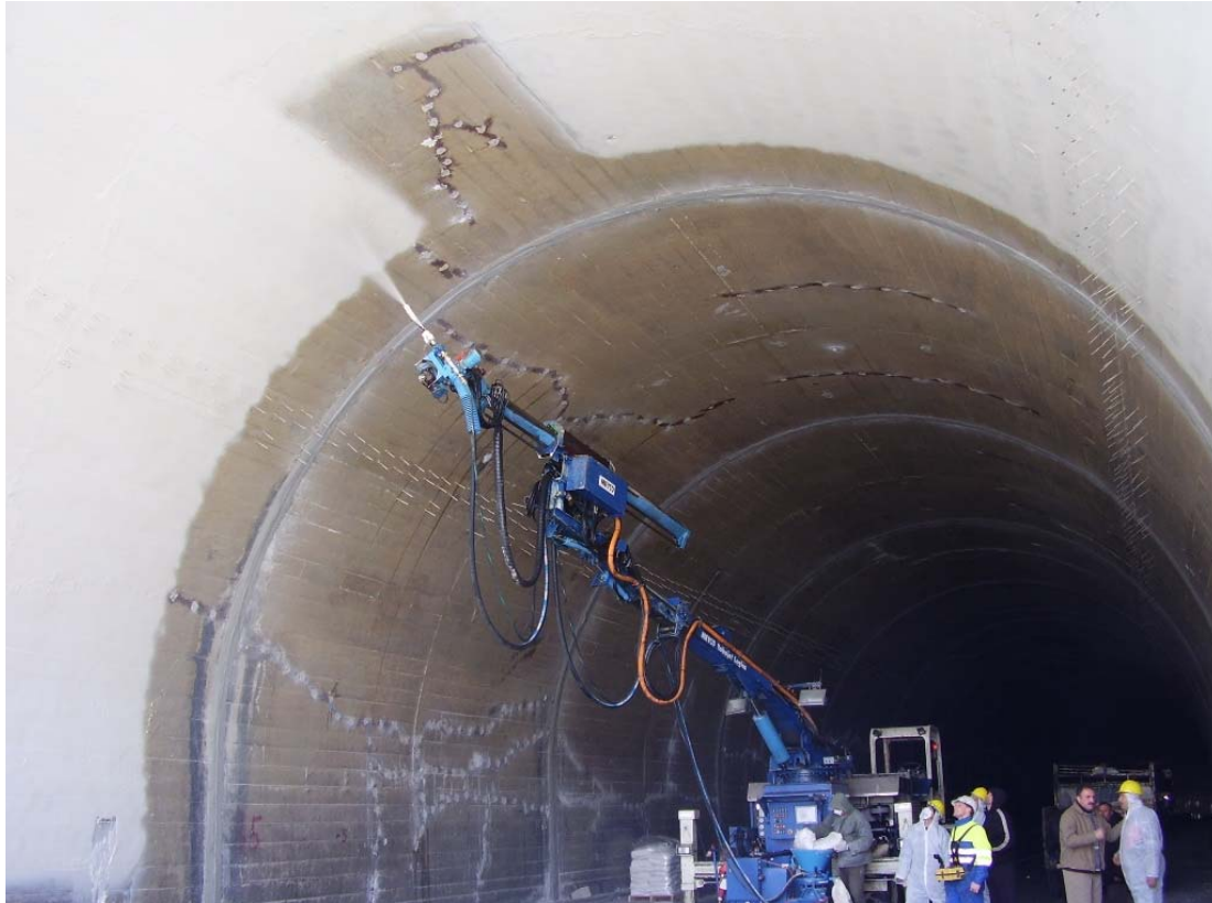
Figure 17. Installation of the Sprayed Membrane. Also Shown Are the Repaired Cracks in Original Lining.
