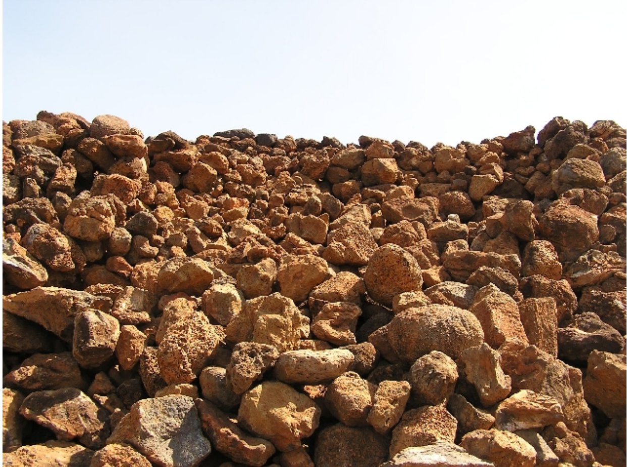
Figure 57. Location 29, slump failure in high rock wall of Pu'ukoholā heiau, west side. See 3-D stereo images of Figure 58 and Figure 59.
