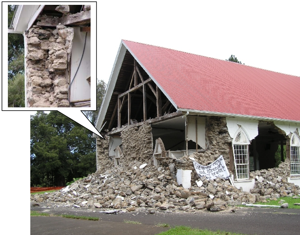
Figure 42. Location 21, Kalāhikiola Congregational Church, Kapa 'au. Weakly cemented stacked rock walls (inset) failed dramatically.
