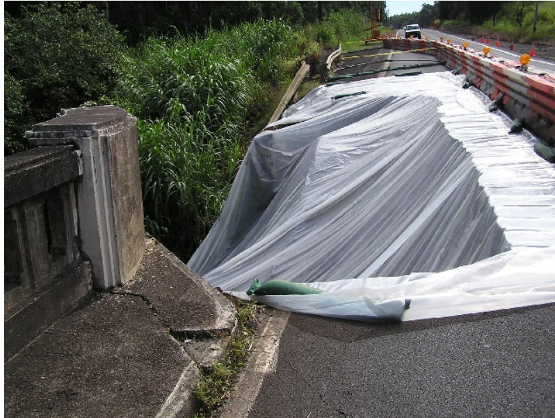
Figure 61. Location 6, Mile Post 35, Hwy 11 near Pa’auilo. Failure of fill at east side of southern approach to bridge.
