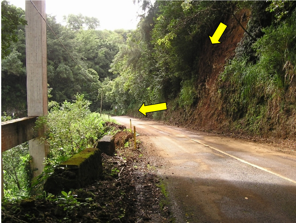
Figure 25. Location 4, old Hwy 11 near Ōōkala, Modern Hwy 11 viaduct above. As evident from red stains in road, soil failed onto and across across Road (arrows) from very steep road cut; typical of many such slides along this road.
