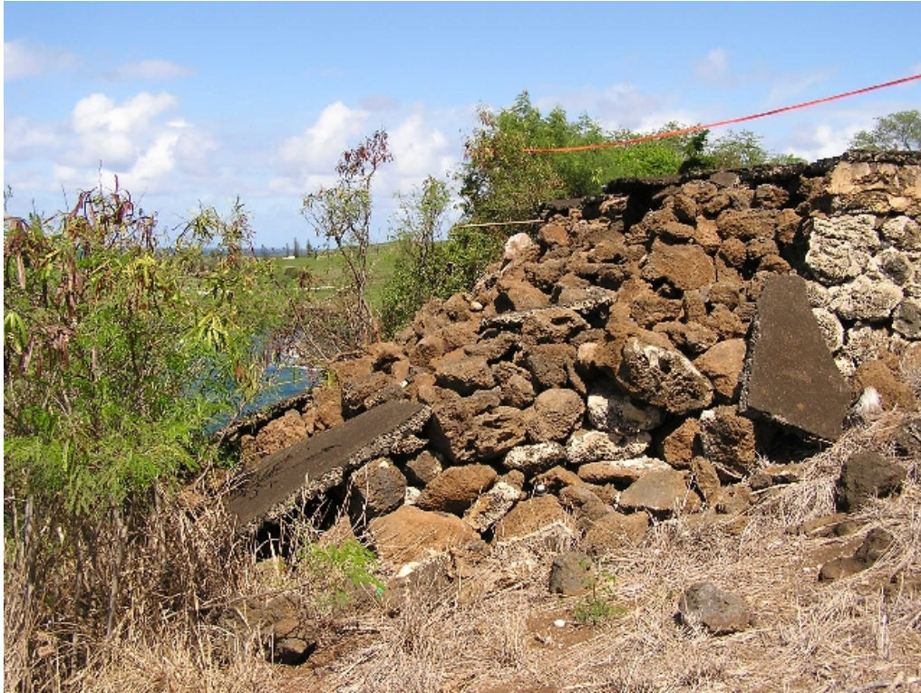
Figure 45. Location 23. Collapse of dry stacked rock wall supporting paved parking area for shoreline access at Puakea Ranch end of trail to Honoipu Landing, due to cliff failures undermining wall foundation.
