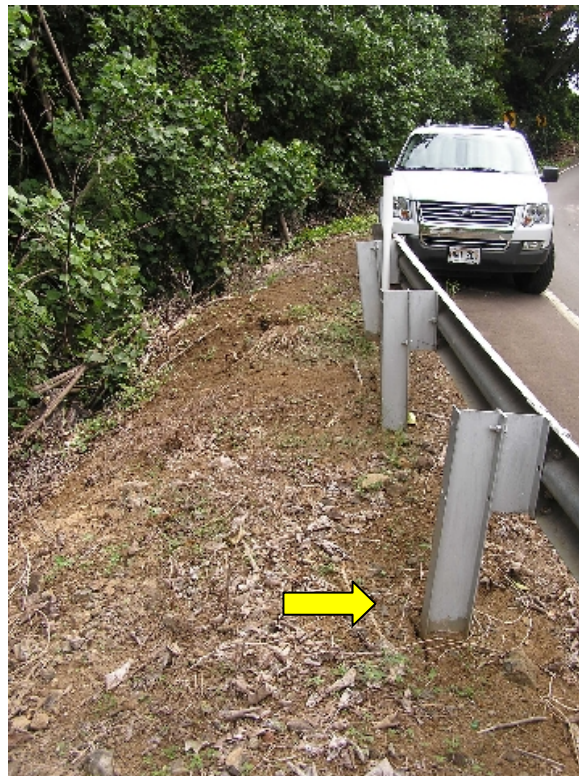
Figure 63. Location 18, Hwy 270 near Makapala, down slope side. Arrow indicates tension cracks and short head scarp 30 cm high at crest of steep and high fill slope.
