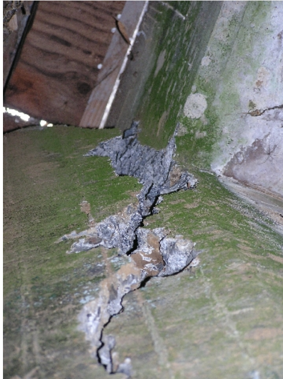
Figure 66. Location 20, bridge at approximately Mile Post 28, Hwy 270. At SW corner of bridge, looking upward at wooden plank sidewalk above. Fresh spalling of bridge abutment headwall at old, pre-existing cracks.
