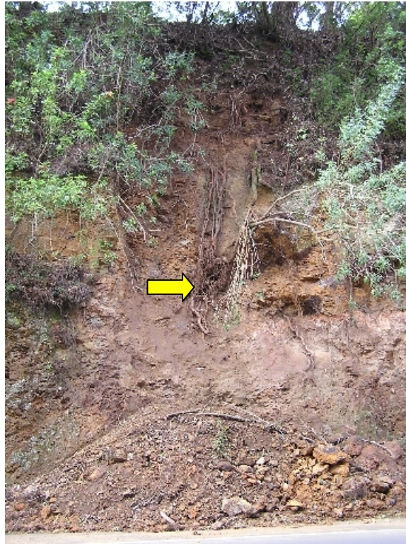
Figure 27. Location 16, Near Kapa'au (Kohala), Hwy 270. Tree roots (arrowed) within relict rock mass fractures degraded the stability of road cuts in soil.
