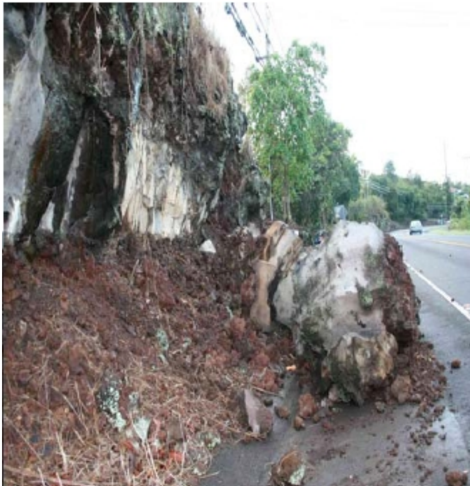
Figure 8. Failed rock cut: massive a'a block undermined by raveled a'a clinker (Chock, 2006; after Robertson et al, 2006).
