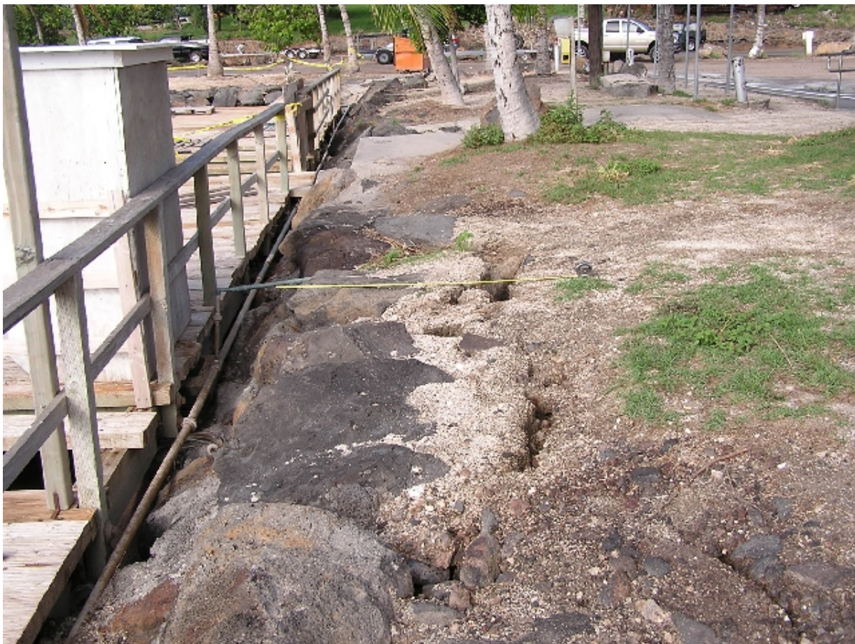
Figure 38. Location 27, Kawaihae Small Boat Harbor. Lateral spreading, and damage to dock. Liquefied sand was ejected from the ground crack (white sand).
