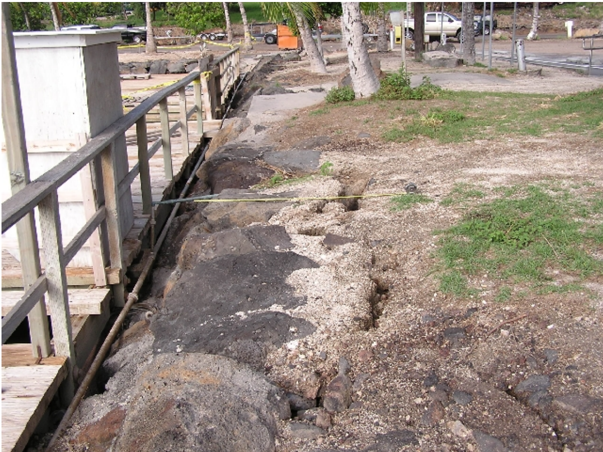
Figure 38. Location 27, Kawaihae Small Boat Harbor. Lateral spreading, and damage to dock. Liquefied sand was ejected from the ground crack (white sand).
