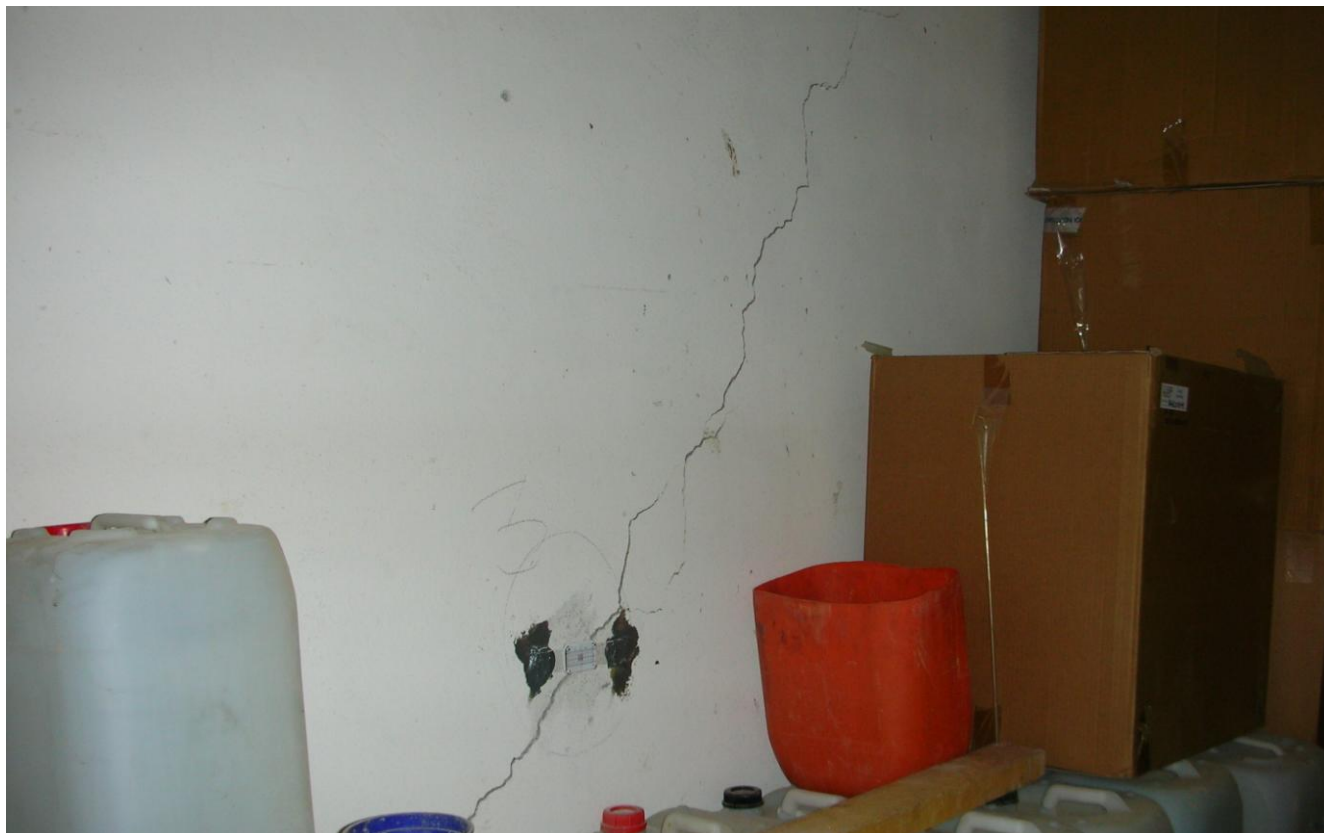
Figure 2. Wall damage inside the warehouse.
