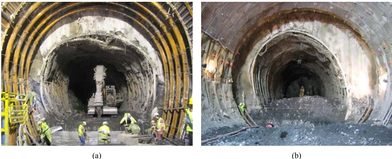
Figure 1. Squeezing rock reduces the tunnel cross section in the Saint Martin La Porte access adit (Lyon-Turin Base Tunnel). The photographs show re-mining works needed in order to cope with the difficult conditions encountered.
