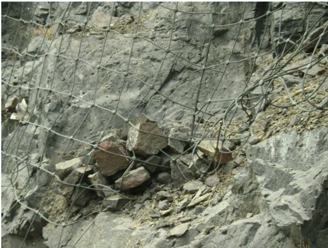
Figure 9. Trapped rock blocks at the toe of the slope.
