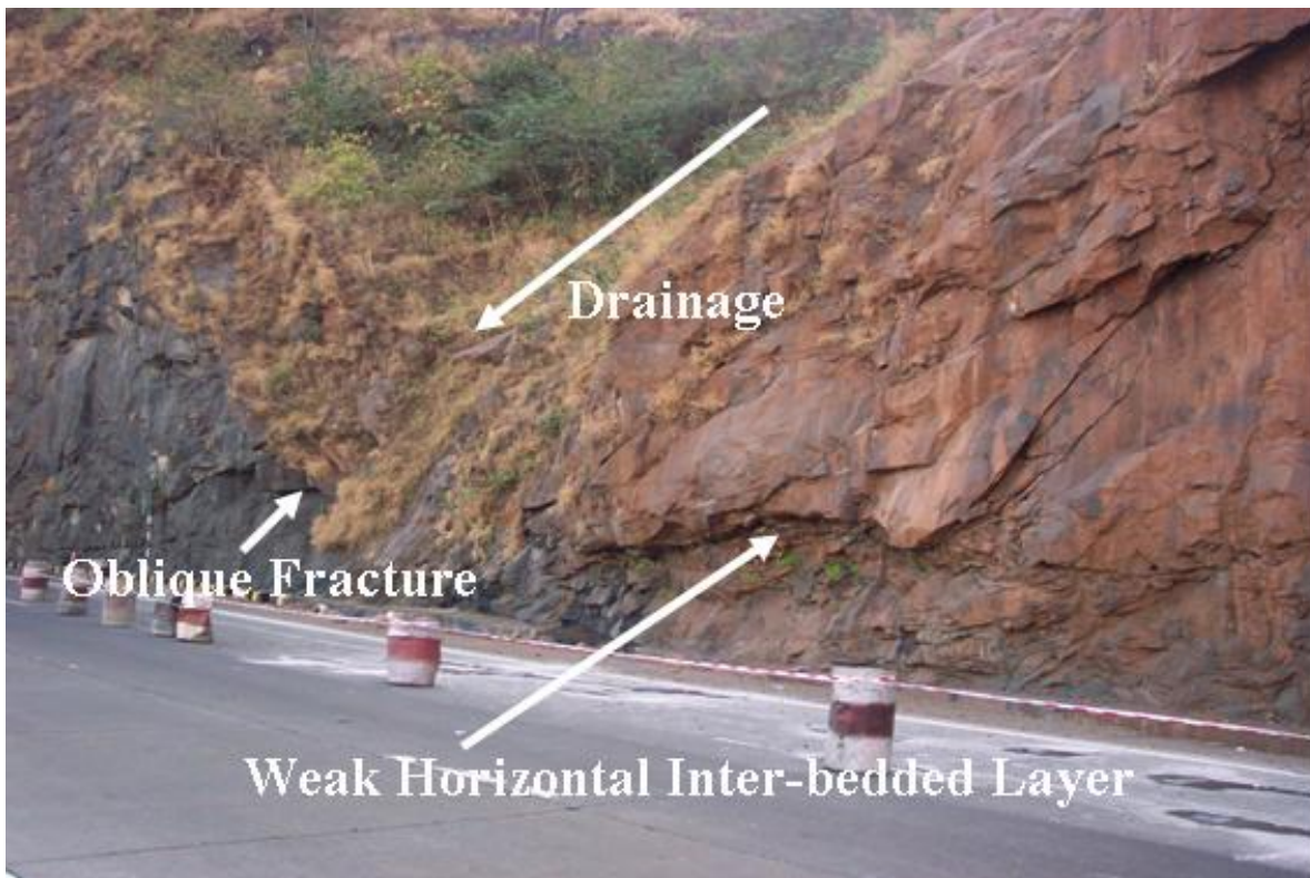
Figure 6. Intersection of oblique and sub-horizontal fractures.
